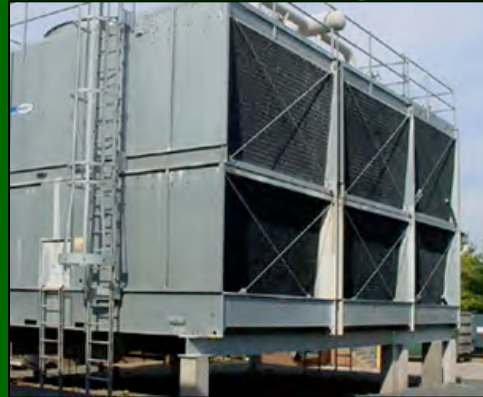
Cooling Tower Water Recycling
