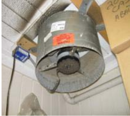
Exhaust fan open to attic (below)
