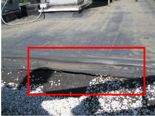
Membrane de-lamination where old and new roof membranes meet
