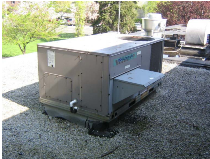
Packaged Rooftop HVAC Unit on West Side First Floor Roof
