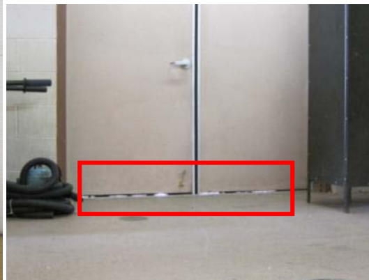
Missing/worn weather-stripping along bottom of exterior door in main garage area
