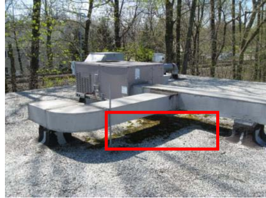
Uncontrolled mold growth on roof, indicating standing water
