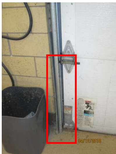
Worn weather-stripping; light visible through garage door
