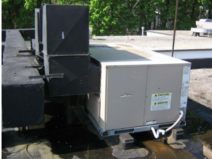
Cooling Only Rooftop Unit Serving the Second Floor Offices
