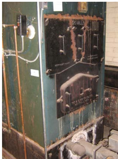
Gas-fired Hot Water Boiler, Converted In 1990
