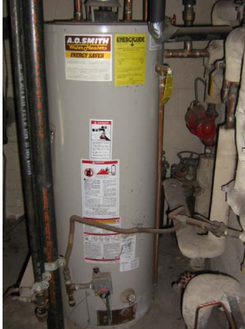
Gas-fired Domestic Water Heater in Boiler Room
