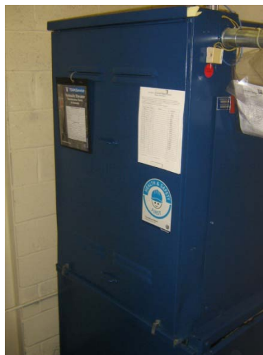
Elevator Hydraulic System
