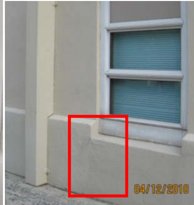
Cracking of exterior finished around window
