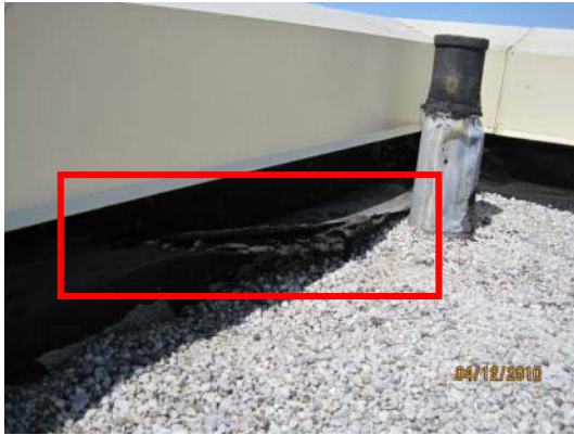
Sagging roofing material at parapet wall
