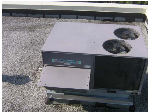
Packaged Rooftop HVAC Unit
