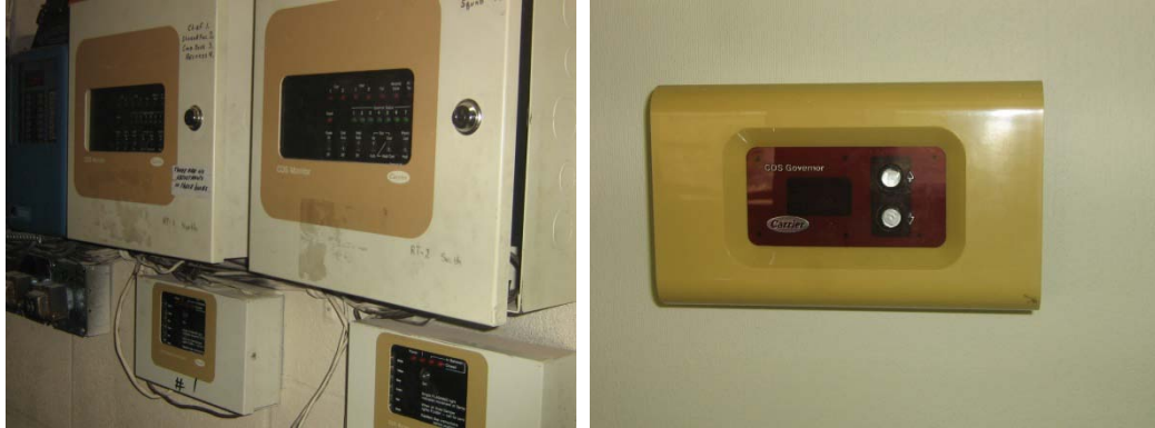
Automatic Temperature Control System Components, Including Thermostat with No Reading (not operational)
