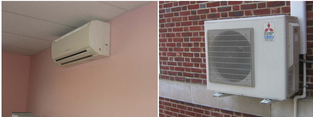
Split System Heat Pump Evaporator (left) and Condensing Units
