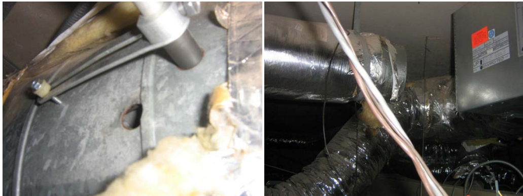
Ductwork penetration (left) and open ductwork near zone damper
