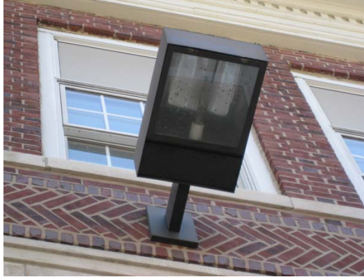
Metal Halide exterior light
