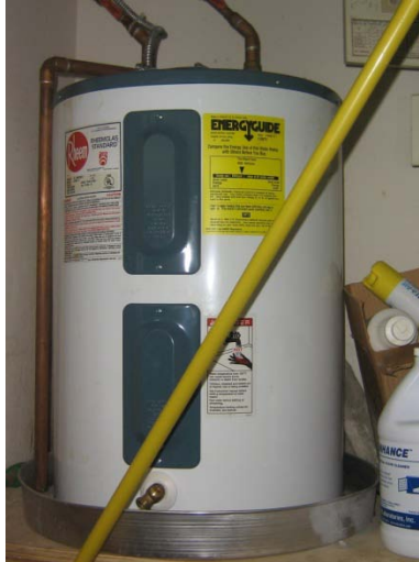
Electric Domestic Water Heater in Main Level Janitor's Closet
