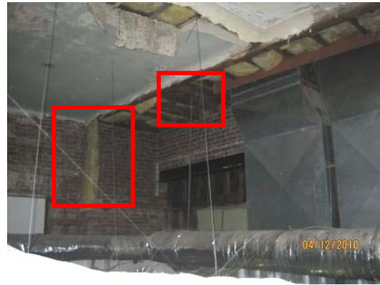
Uneven/missing attic insulation found above deteriorating, original plaster ceiling
