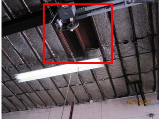
Sections of missing ceiling insulation found, Mechanics Garage
