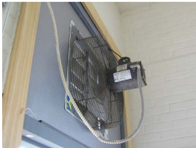
Typical Louvered Exhaust Fan Above Pump House Door
