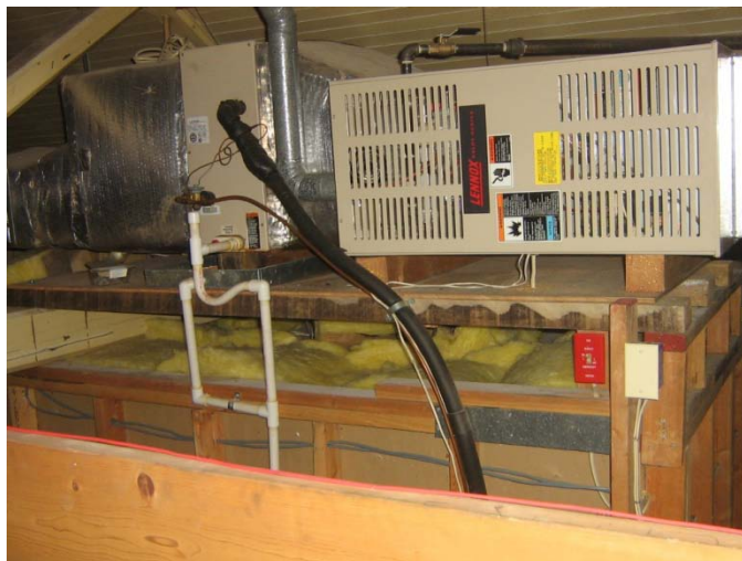
Heating & Cooling Split System Air Handling Unit in Attic Above Locker Room
