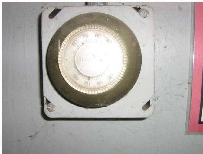
Example of Manual Thermostat, Located in the Main Office and Garage Building
