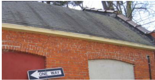
Signs of mold/water damage on roof shingles
