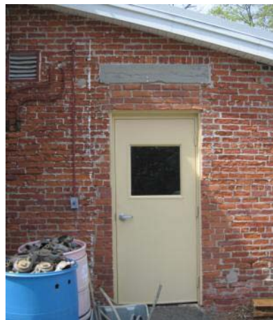
Efflorescence on brick and masonry walls indicate moisture presence within the wall cavity.
