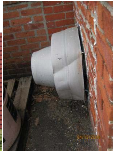
Fan not properly installed on wall surface
