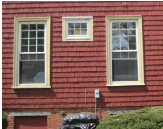
Damaged/cracking exterior wall finishes
