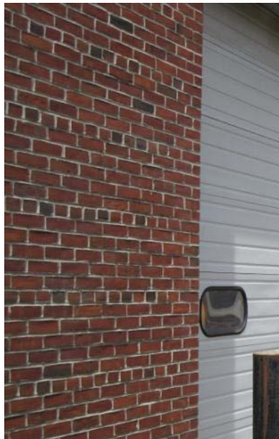
Cracked/deteriorated bricks and mortar joints
