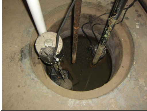
Submersible Sump Pump In Garage
