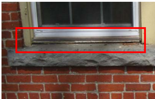
Cracked or aged caulk around frame/sill on the exterior
