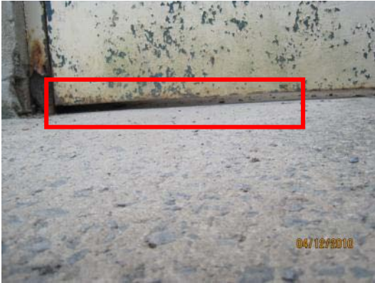
Exterior aluminum door not properly sealed, Mechanics Garage
