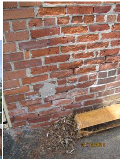
Cracked/deteriorated bricks and mortar joints
