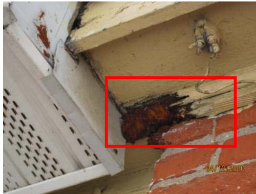
Insect nesting in roof cracks and cavities
