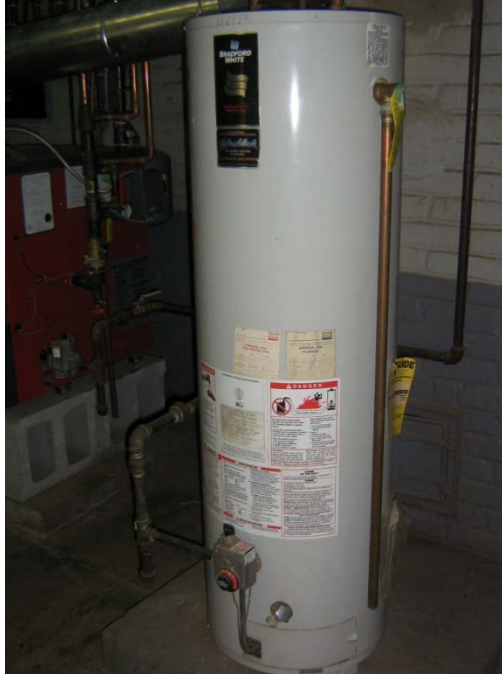
Gas-fired Domestic Water Heater in Front Garage
