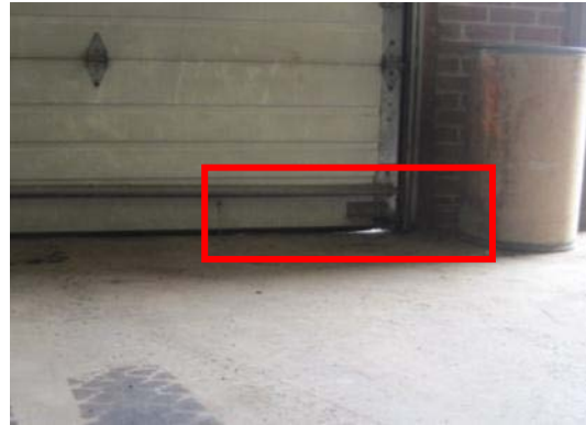
Garage door not properly sealed, Middle Garage
