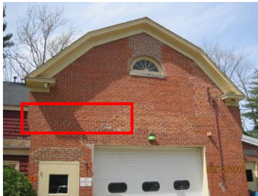
Cracked/deteriorated bricks and mortar joints
