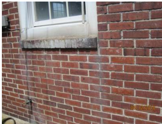
Exterior mold/water damage signs on areas around windows
