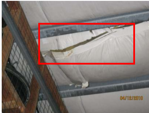
Uneven attic insulation found in some areas, Left Garage
