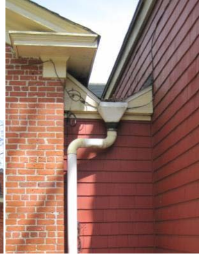
Severely clogged gutters
