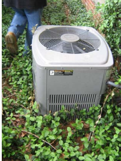
Separate Air-cooled Condensing Unit Located on Grade
