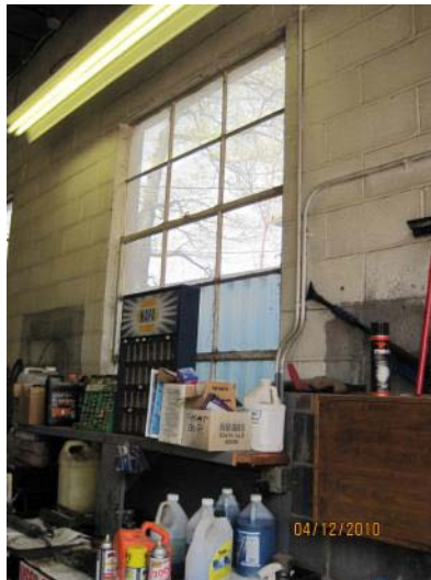
Single-glazed window with ineffective frame
