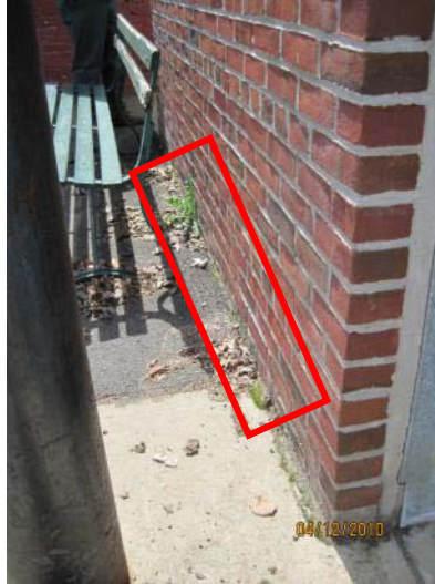
Vegetation growth at base
