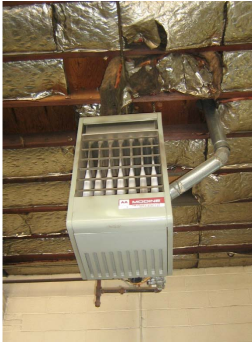
Typical Gas-fired Unit Heater in the Corner of Each Main Garage Section
