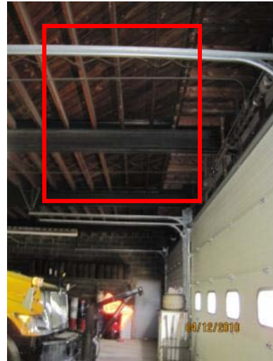
No insulation at all despite being a conditioned space, Middle Garage
