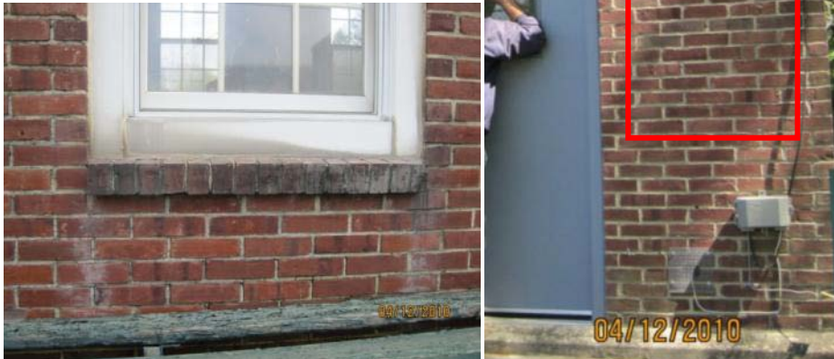
Well House Wall Water Damage and Infiltration
