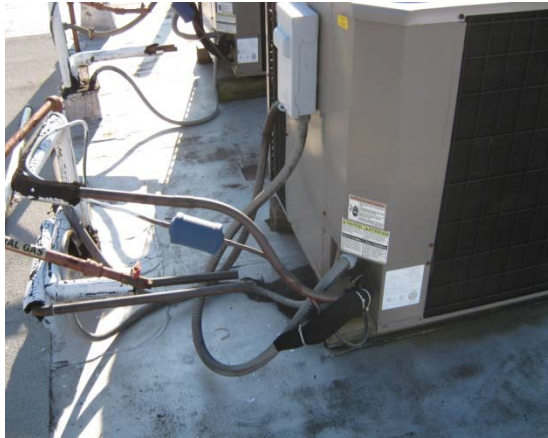
Photo showing broken or missing insulation on Refrigeration lines.
