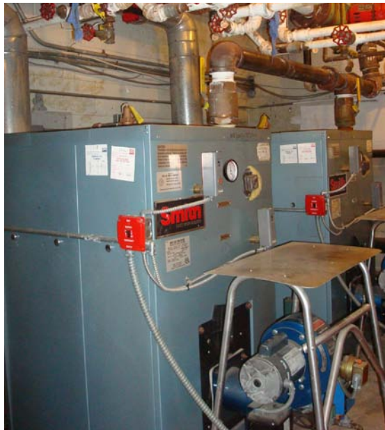
Smith Hot Water Boilers in Basement Boiler Room
