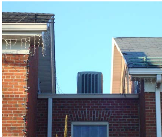
Rooftop Condensing Unit Serving 2003 Addition Area (left)
