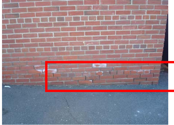
Brick façade, back corner of Police Department in need of re-pointing
