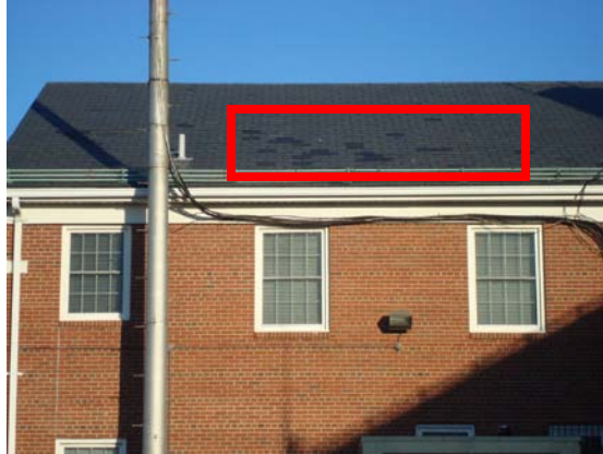
Damaged/replaced roof slate tiles
