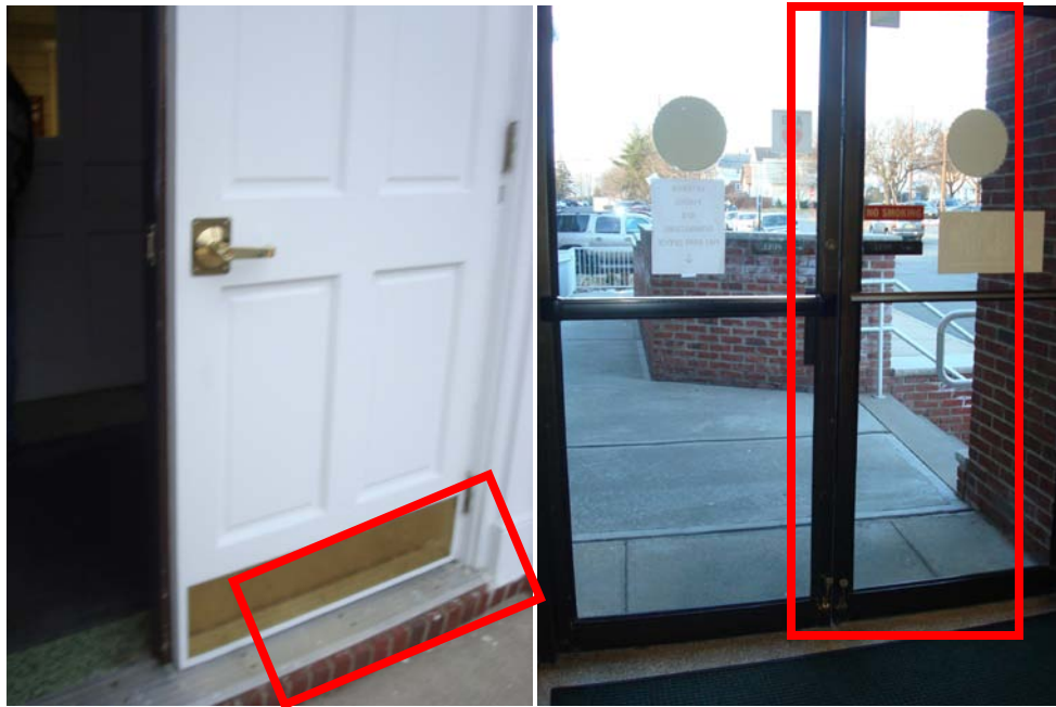
Door weather stripping needs to be checked on regular basis
