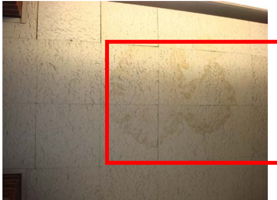
Water stains on ceiling tiles
