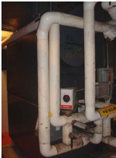
AC-1 Basement Boiler Room with HW & Glycol Coils
