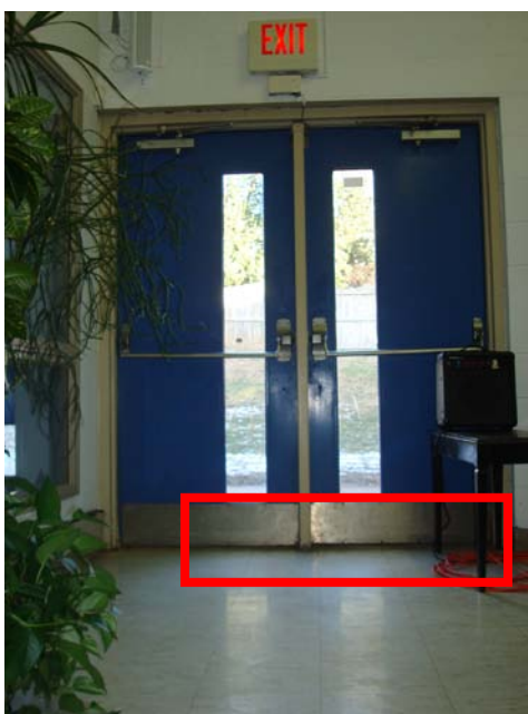
Doors in need of weather-stripping
