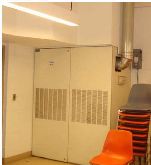
Airedale Closet Furnace in Exercise Room, with flue piping
