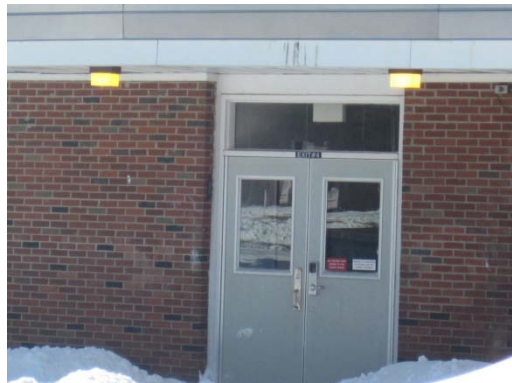
Exterior lights left on during daylight hours
