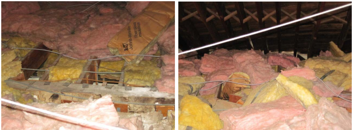
Fiberglass insulation haphazardly displaced
