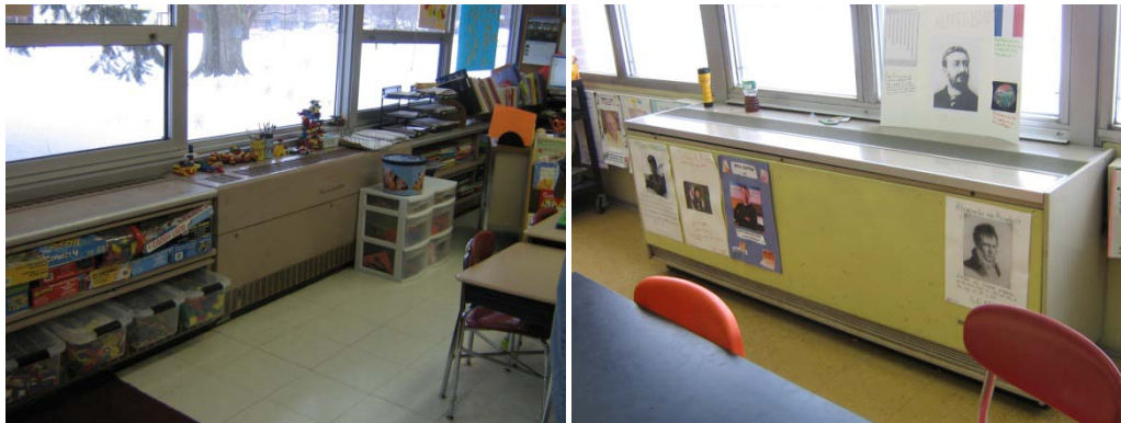
Unit Ventilators in B Wing (Left) and C Wing (Right)
