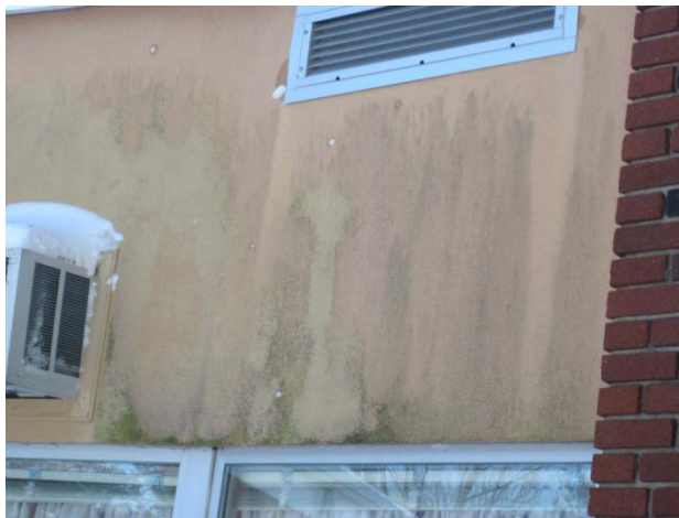
Water damage EIFS
