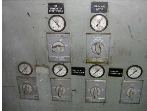
Pneumatic Control System Panel in C/D Wing Boiler Room
