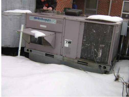
Packaged HVAC Unit on Grade Serving TV Studio
