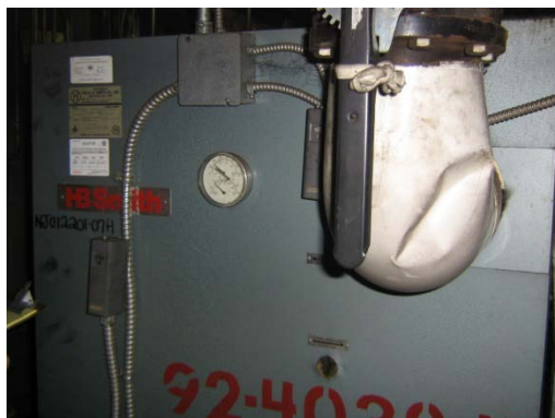
C/D wing boiler
