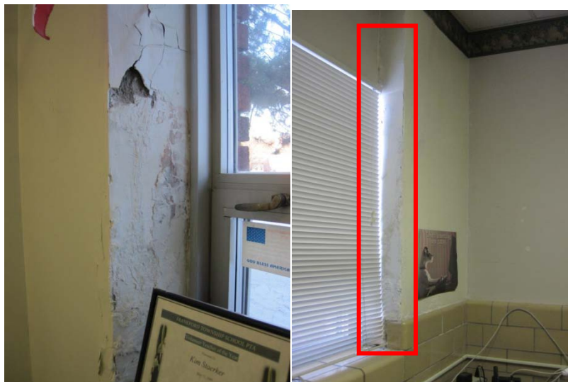
Interior wall finish – lath and plaster wall damage
