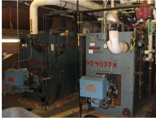
A/B wing boilers
