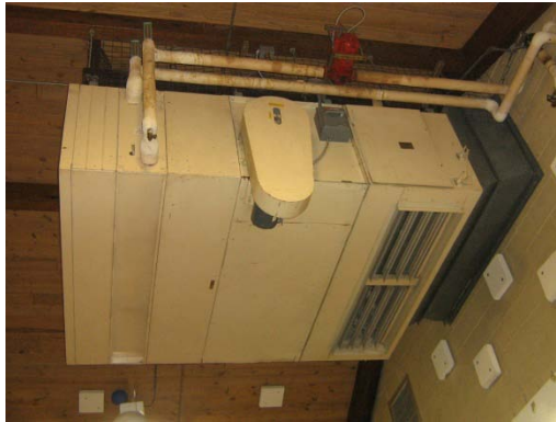
H&V Unit Suspended From Roof in Small Gym
