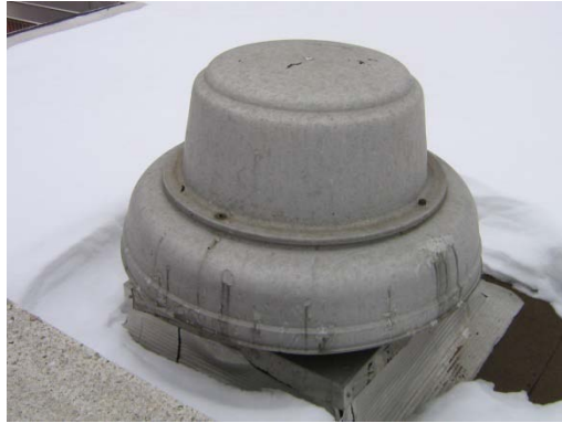
Typical Rooftop Exhaust Fan
