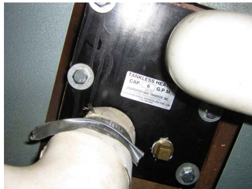
Typical Tankless Boiler Immersion Domestic Water Heater in A/B Boiler
