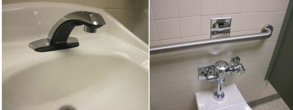
Updated bathrooms with sensors for toilets and sinks (with 0.5gpm aerators)
