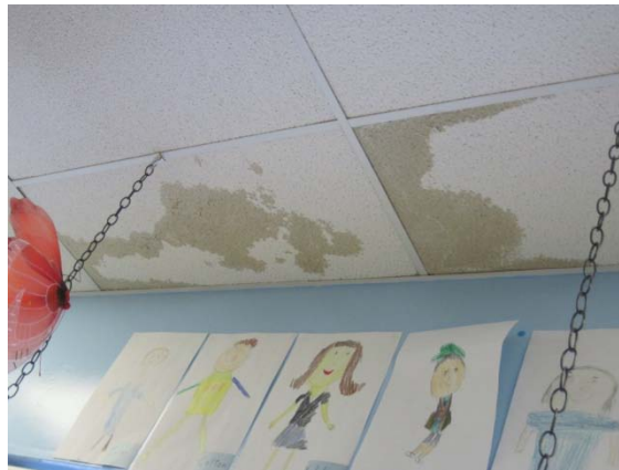
Image showing damaged ceiling tiles in classroom
