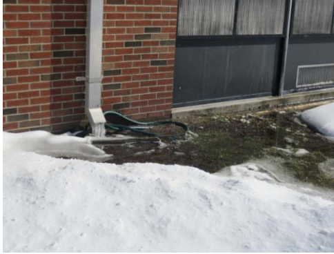
Water pooling at base of building due to extreme weather condition
