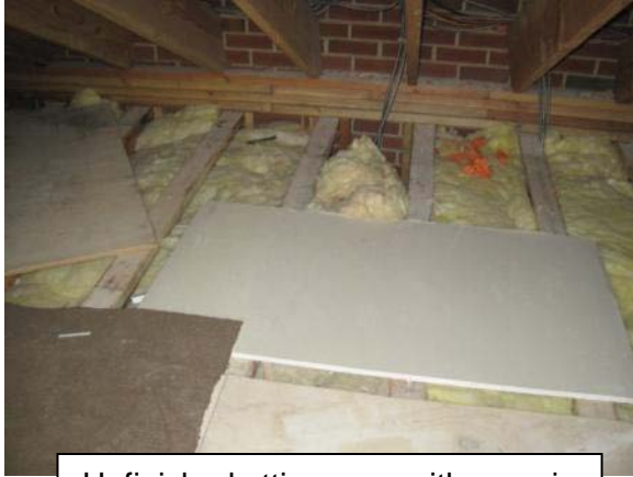
Unfinished attic space with gaps in insulation.
