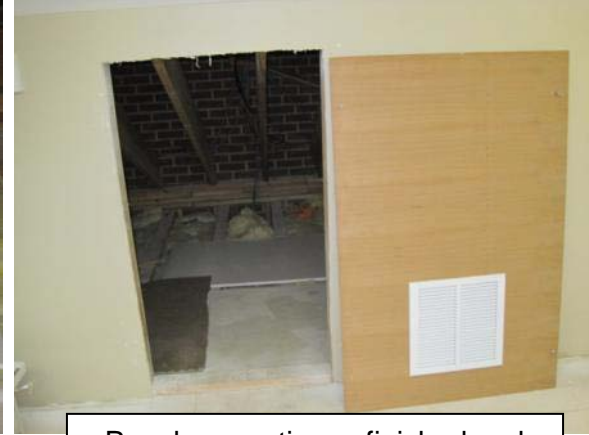
Panel separating unfinished and finished sections of attic which should be screwed in.
