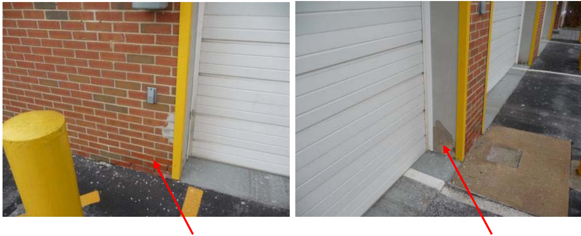
Brick re-pointing and sidewall repairs needed around a couple of the overhead doors
