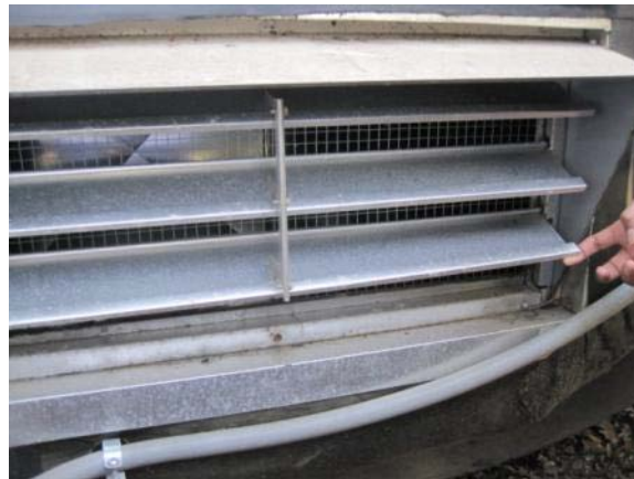
Lennox RTU gravity damper on return duct
