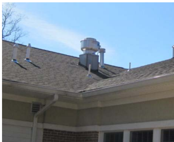
Kitchen exhaust fan mounted on roof
