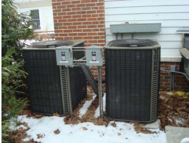
York Condensing units serving Furnace 1 & 2, located outside
