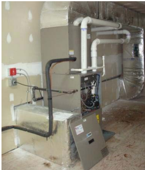
Attic Furnace 2 – 135MB, Condensing Type
