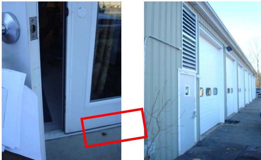
Office door in need of weather stripping; typical garage doors
