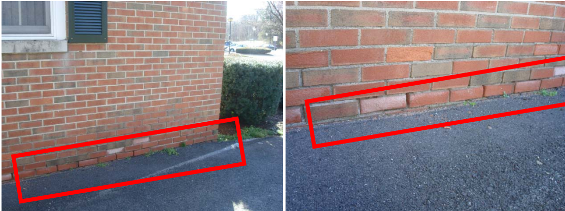
Bottom area of brick façade needing re-pointing
