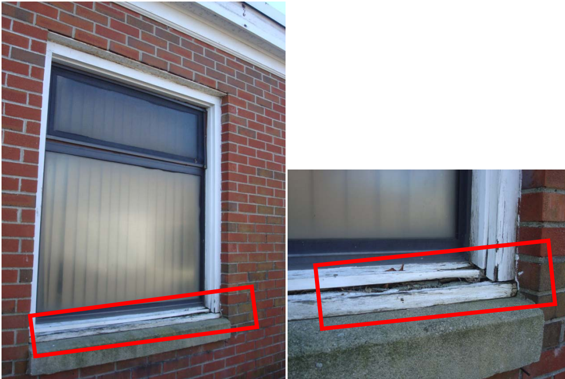
Window lintel needing caulking above it and painting; rotted wood members should be replaced to prevent insect infestation
