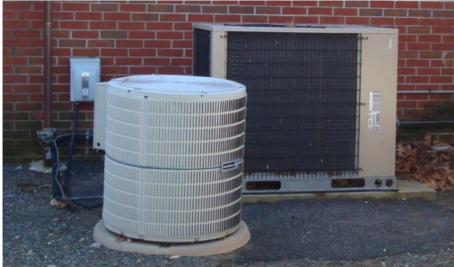
Two condensers installed in back of building
