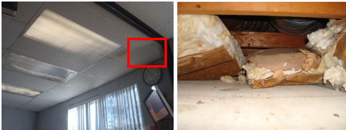
Ceiling tile water stain; Batt insulation above the drop ceiling
