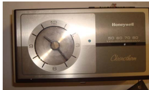
1 st Floor Manual Thermostats (top), Basement manual thermostat (bottom), set at 68°F/70°F
