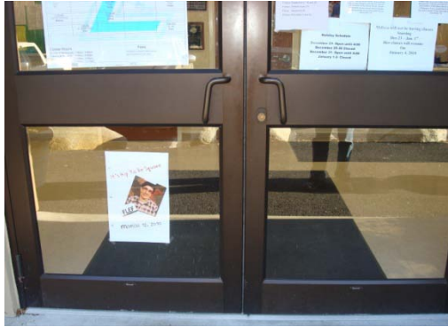
Front entrance doors in need of weather stripping
