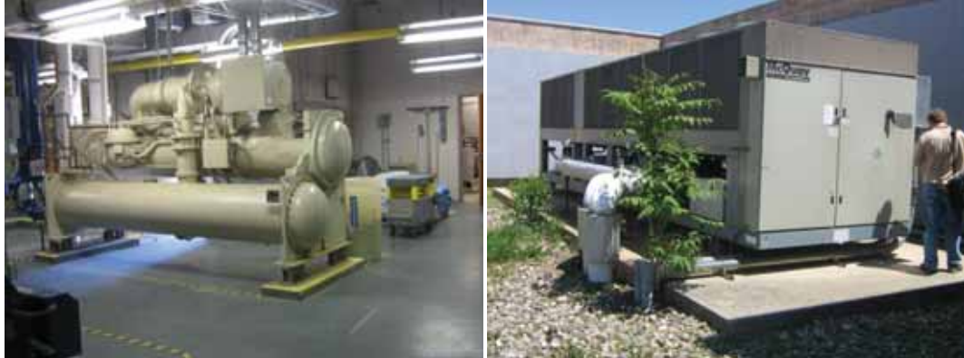
Water-cooled chiller (l.) and air –cooled chiller (r.)
