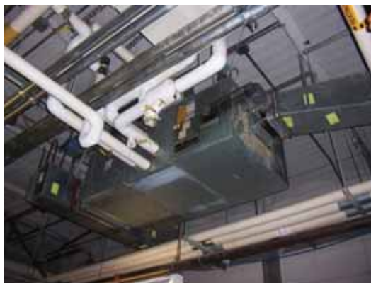
Hot and chilled water air handling unit suspended from roof deck
