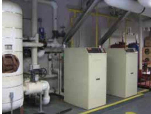
Domestic water heaters
