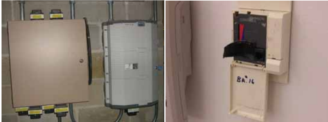
Johnson Metasys control panel (l.) and typical thermostat (r.)
