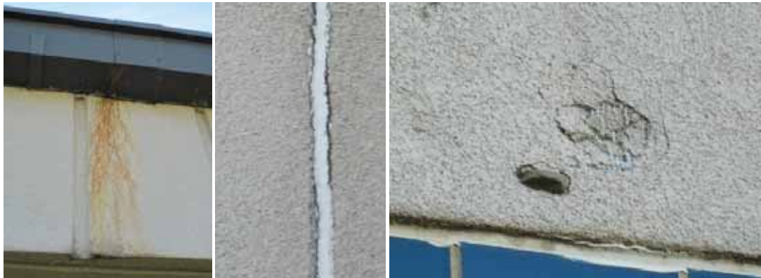
Signs of water damage at perimeter walls due to damage roof flashing or gutters
