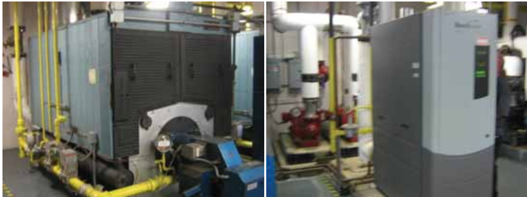
One of three cast iron boilers (l.) and condensing boiler (r.)
