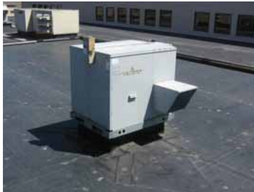
Energy recovery unit above cafeteria
