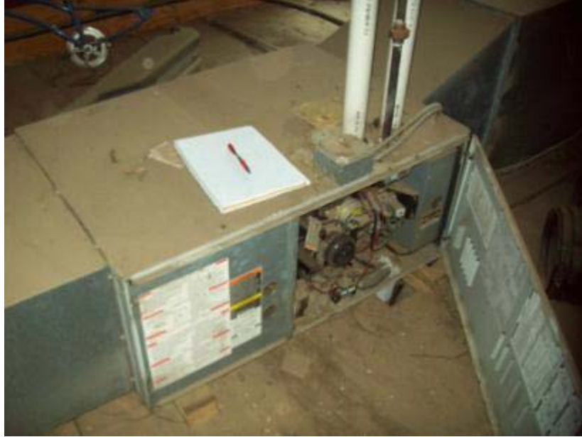
Carrier air handling unit located above office spaces
