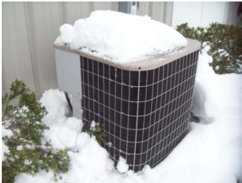
Carrier condensing unit located on front side of building
