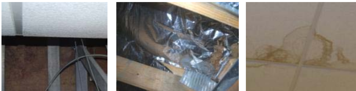
Damaged/missing roof insulation and ceiling tile with water stains
