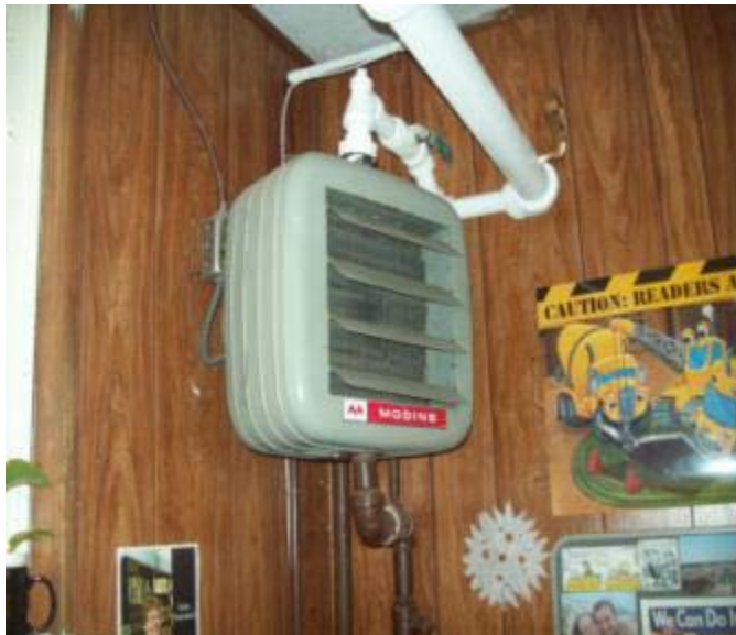
Modine unit heater mounted in Basement level
