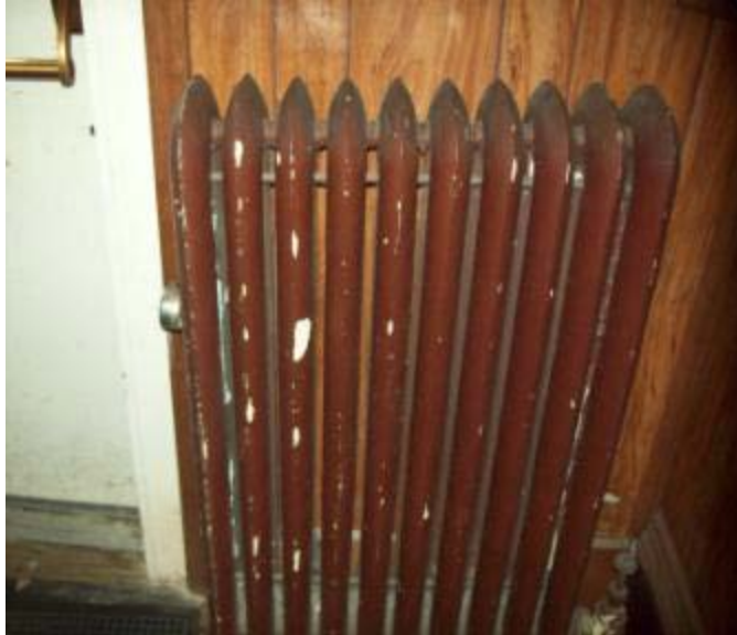
Cast iron radiator located in stairwell
