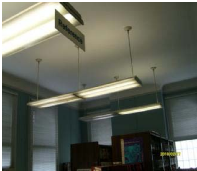
General lighting consisting of T12 fixtures with magnetic ballasts
