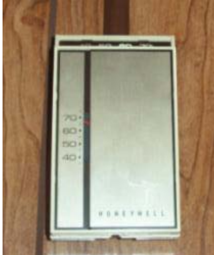
Non-programmable thermostat in Basement
