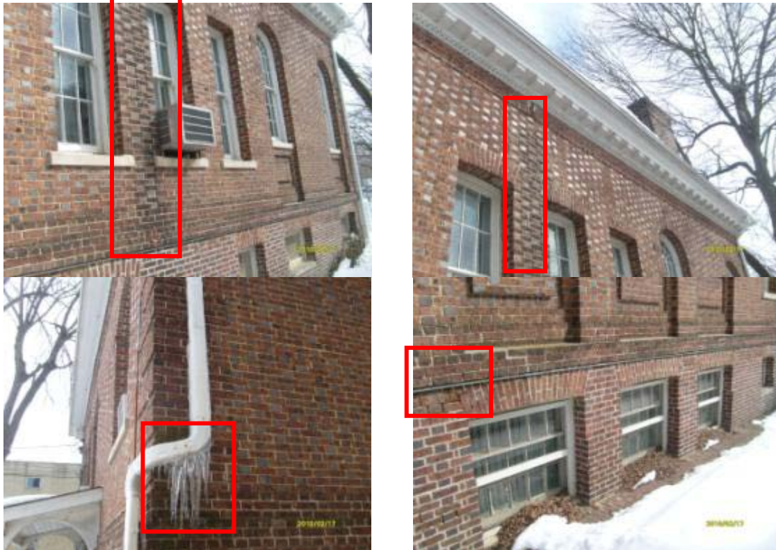
Water damaged brick sections, ineffective downspouts, and sections with missing or deteriorated caulking.
