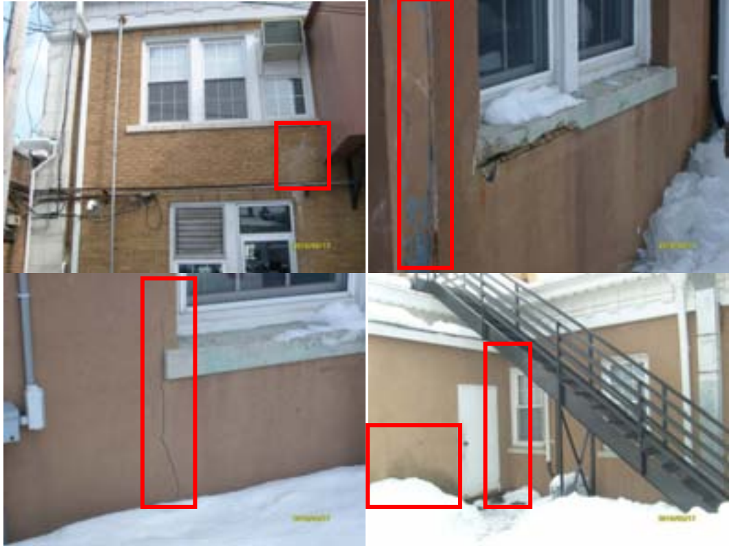
Efflorescence on brick and masonry walls indicate moisture presence within the wall cavity, cracked/aged caulk and damaged exterior wall finishes
