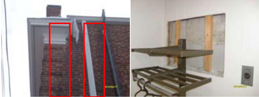
Water damage from uncontrolled roof water run-off due to missing gutters and downspouts (L). Exposed CMU block with no insulation installed (R).
