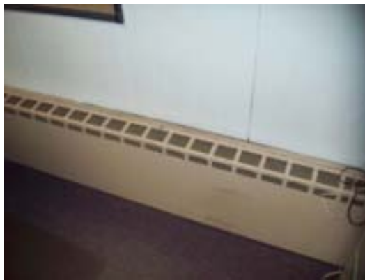
Typical electrical baseboard unit
