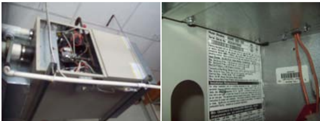
Picture of first floor furnace and nameplate
