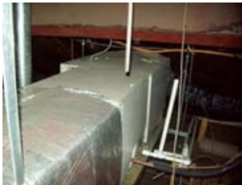
Air handler unit in ceiling plenum
