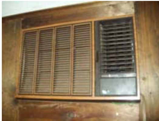
Basement air conditioner
