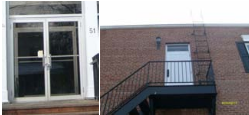
Typical door installations
