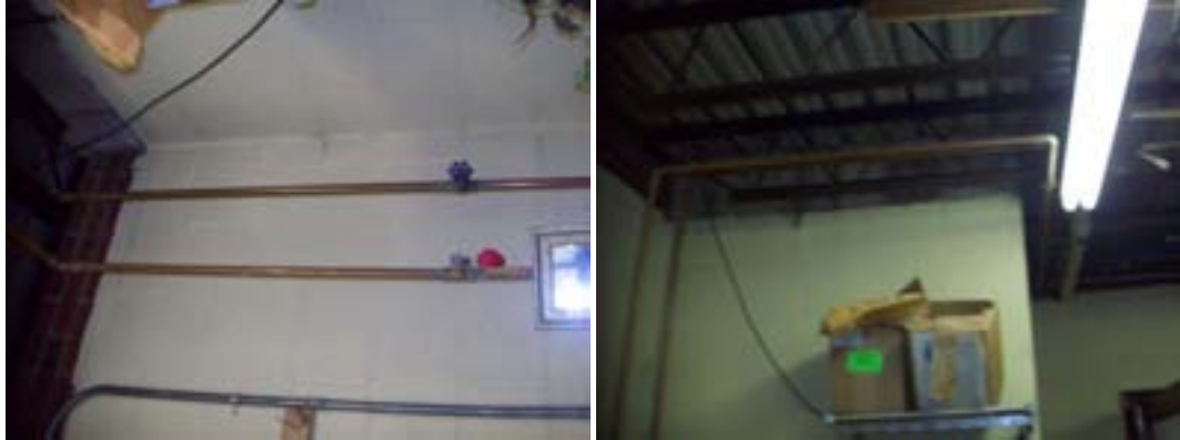
Example of un-insulated copper piping in the Municipal building
