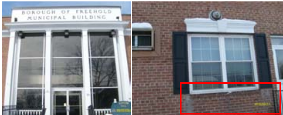
Front of Municipal building, glass entrance area (L). Missing window sill and drip-edge detail (R).
