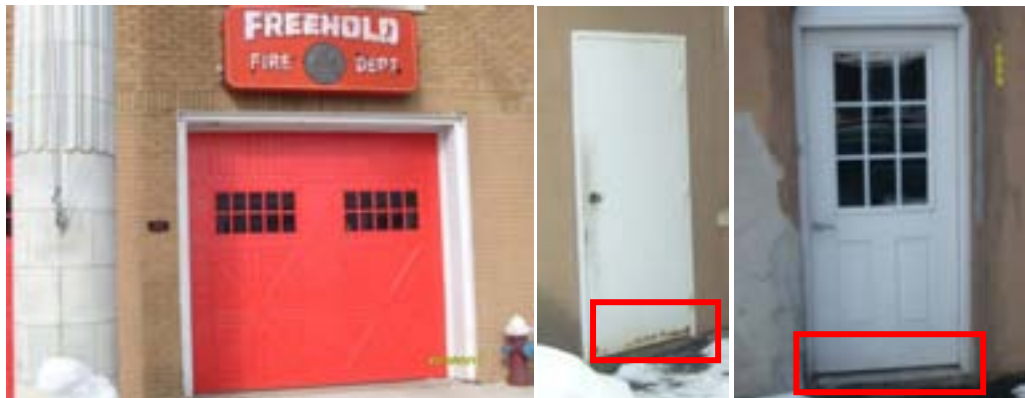
Missing/worn weather-stripping, damaged/warped/aged door frame and exterior mold/water damage signs on areas around doors
