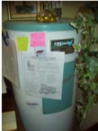
Municipal Building DHW heater
