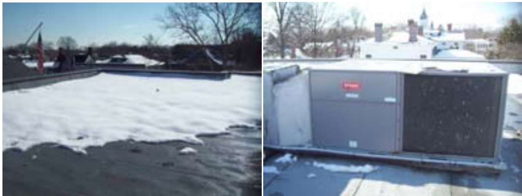
Typical roof installation
