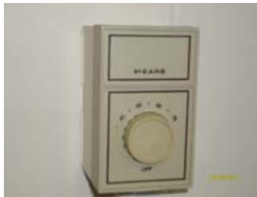
Typical thermostat for electric baseboard units
