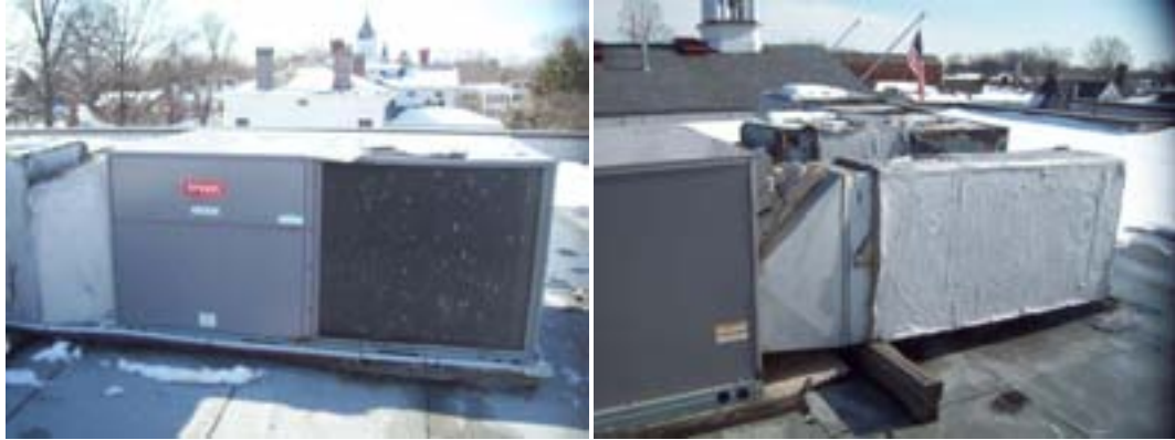
Bryant packaged rooftop unit
