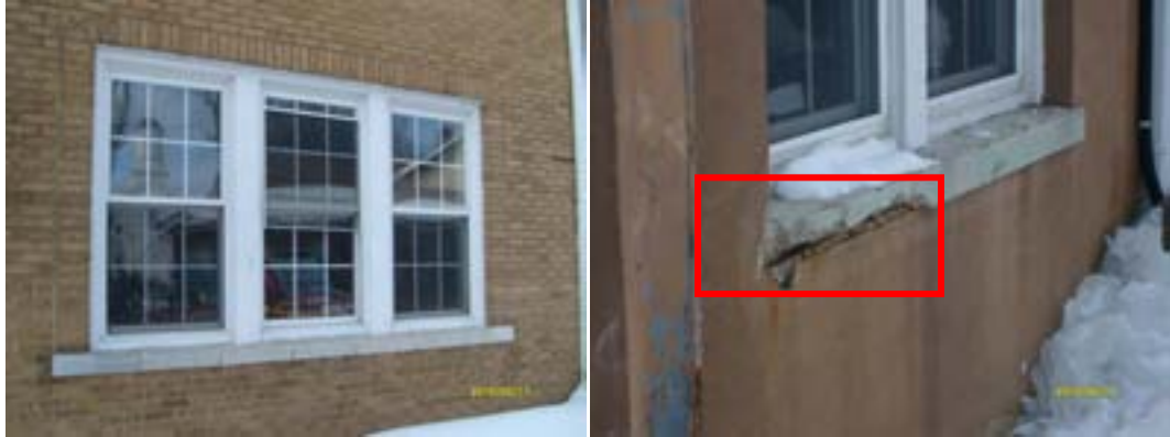
Typical double-hung window (L). Damaged/aged window frame and damaged window sill (R).
