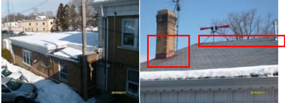
View of lower roof (L). Missing / ineffective flashing and damaged roof shingles on upper roof (R).
