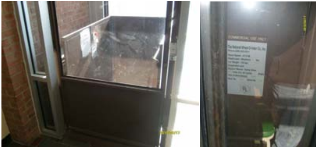
Accessibility lift and nameplate
