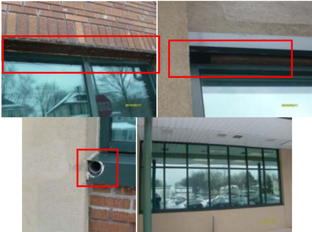
Damaged and exposed window frames that form thermal bridges, warped frames that lead to infiltration, un-insulated conduits that run through windows and a window installation.
