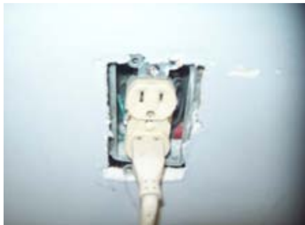
Electrical outlet allowing heated air to be lost to bike storage area
