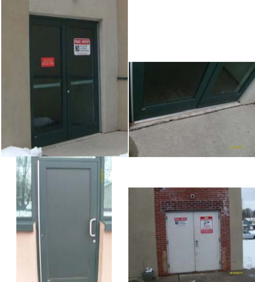
Examples of typical doors with damaged frames, and missing weather-stripping.
