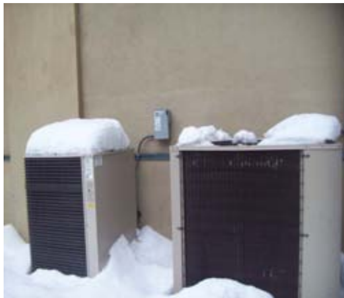
Two of the six heat pumps located on the exterior of the building
