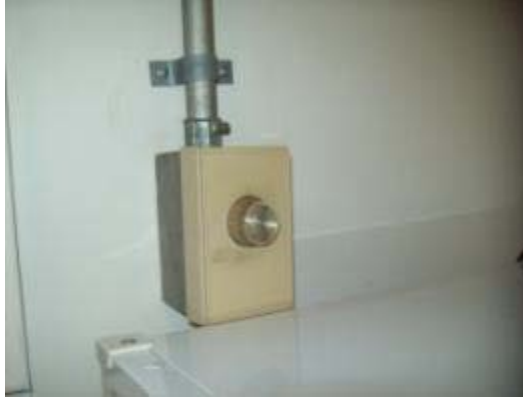
Typical non-programmable thermostat control
