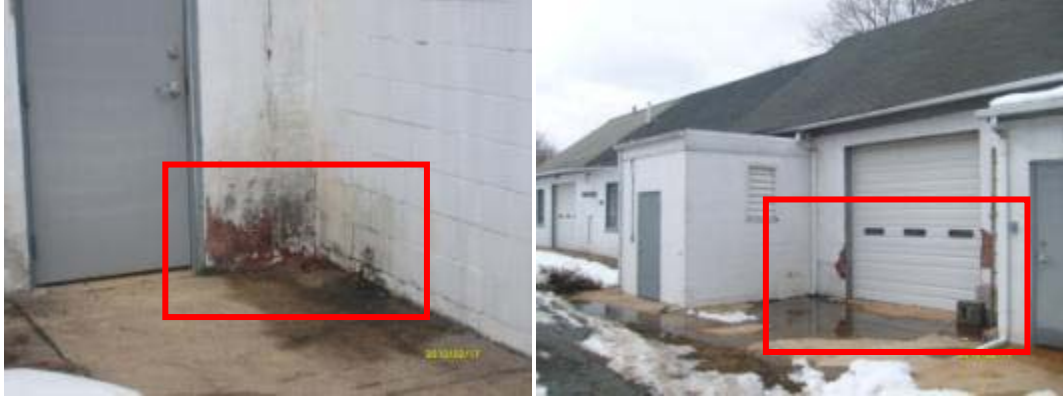
Example of poor site drainage and cracks at exterior surfaces due to water damage
