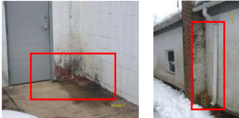
Example of sections with signs of water damage, cracked caulking, damaged bricks and shifted blocks.
