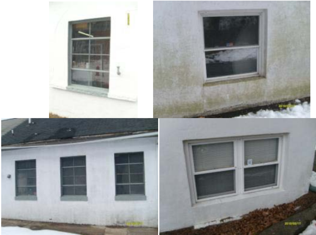
Typical Window Installations with some signs cracked window sills and water damage along frames.
