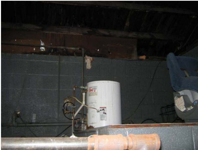
Rheem electric water heater (police garage)
