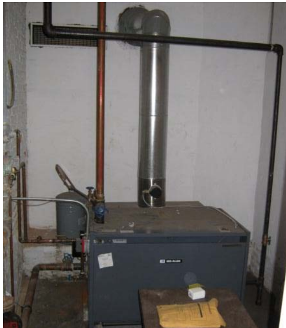
Weil-McLain boiler (former community center)
