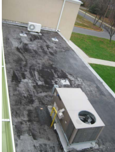
EMI split-system (left) & York RTU (right)
