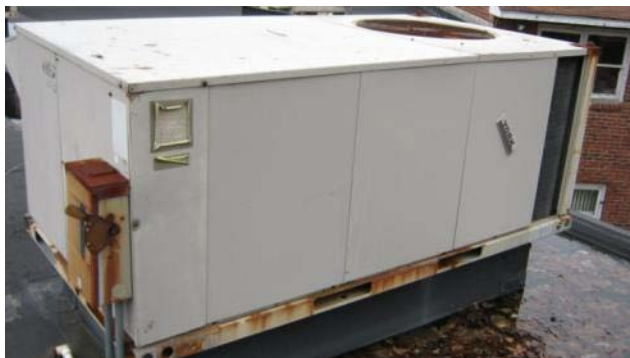
Ponding in bottom-right corner
