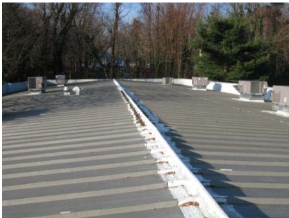
Rooftop Heat Pumps
