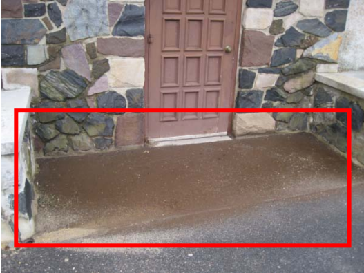
Signs of water pooling around doors and flooding into building
