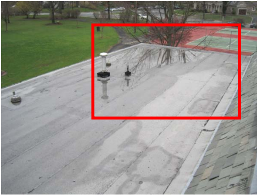
Ponding of water on flat roofs
