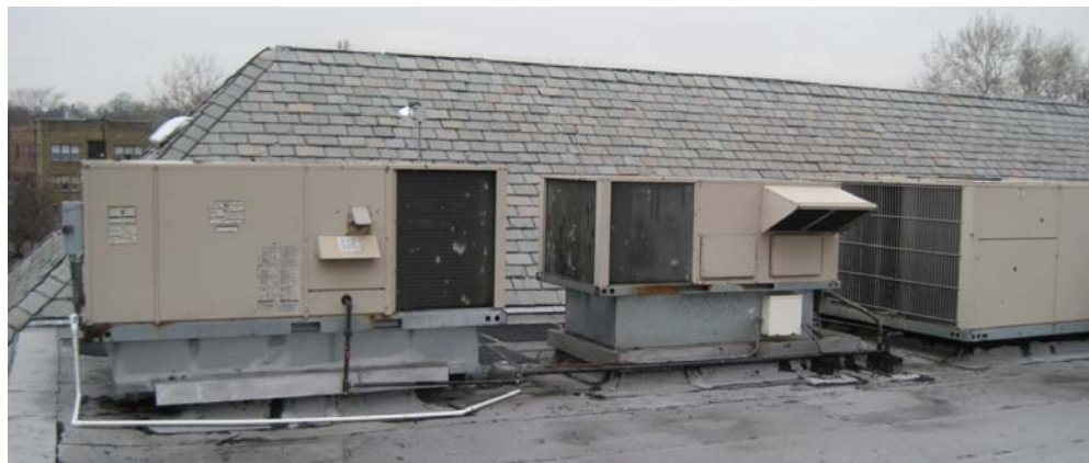
Gas fired DX cooled rooftop packaged units
