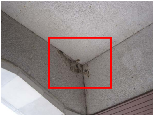
Insect nesting in exterior wall cracks and cavities
