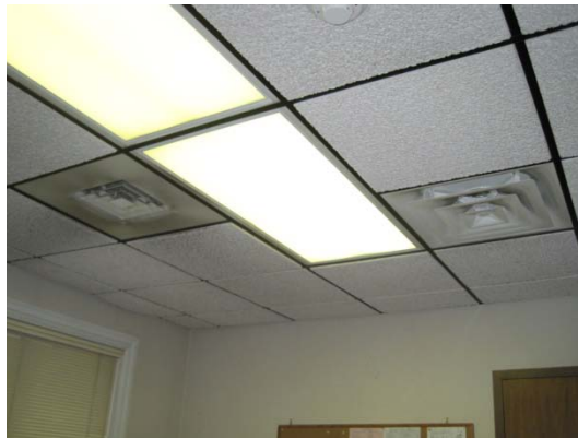
Example of typical fixture with inefficient 4'T12 bulbs and magnetic ballast
