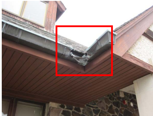
Damaged gutters in the front of the building
