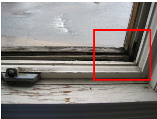
Attic window with missing pane of glass and interior water damage causing window not to operate properly
