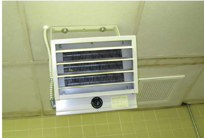
Kitchen electric heater – manual knob control
