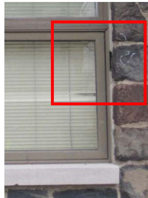
Cracked caulk around frame on the exterior
