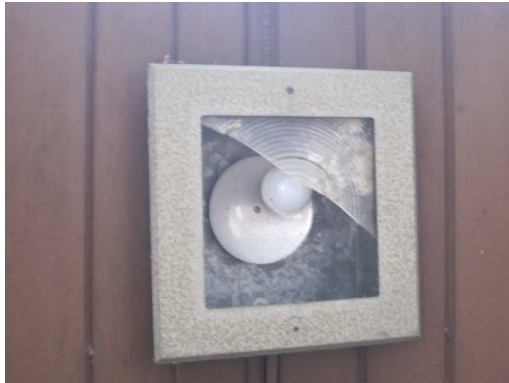
Exterior light fixture with inefficient incandescent bulb and damaged lens
