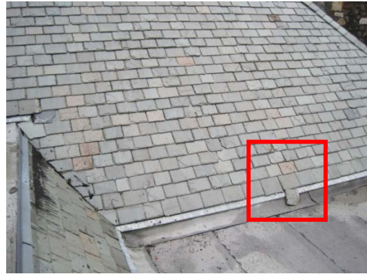
Loose slate shingles
