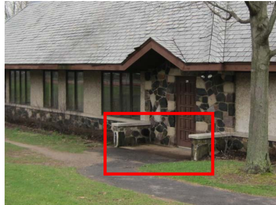
Image showing area of water pooling near exterior door
