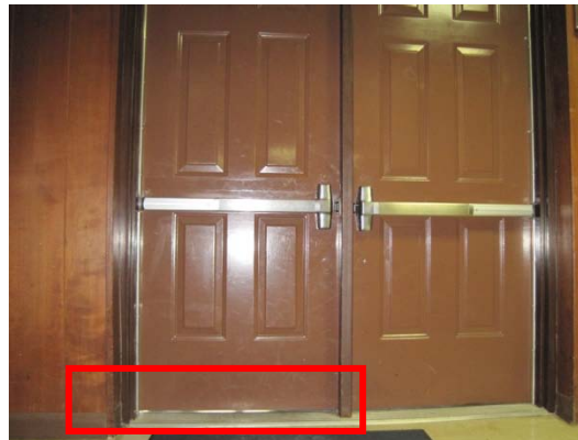
Missing and worn weather-stripping around doors
