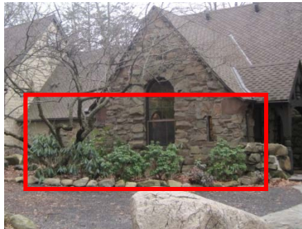
Ground vegetation allowed to grow against exterior wall surfaces could cause damage to building
