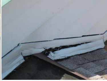
Wood rot due to proximity of water runoff from roof
