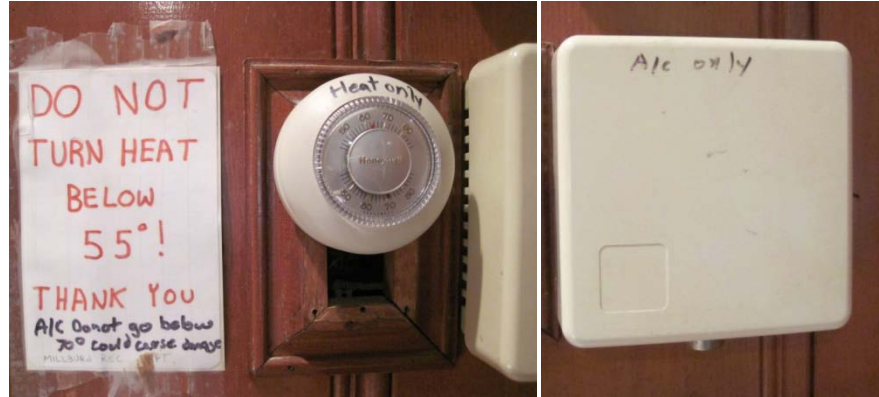
Controls for heating and cooling in Gero Park building
