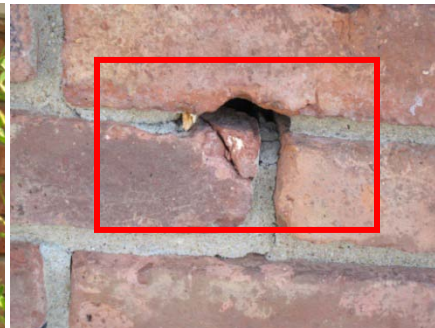
Damaged brick on exterior wall
