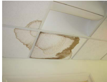
Water damaged ceiling tile
