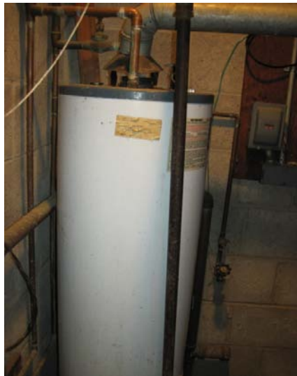
DHW tank in mechanical room
