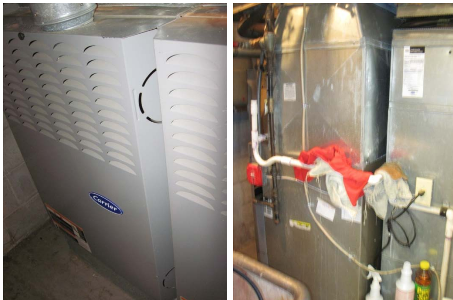
Gas-fired furnaces in mechanical room at Gero Park
