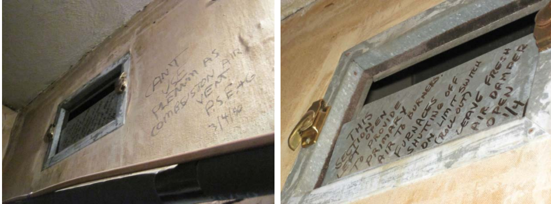
Sheet metal cut off of return plenum to allow needed fresh air for combustion
