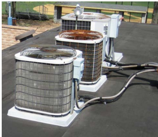
Three condensers on flat roof section
