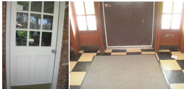
Missing and worn weather-stripping around and between doors allows air to infiltrate into building
