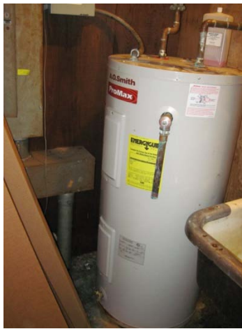
Water heater in closet
