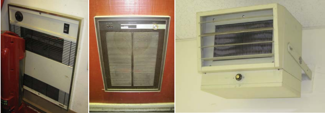
Electric heaters serving bathroom and office area
