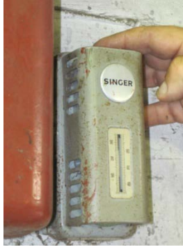
Control for electric heater in garage
