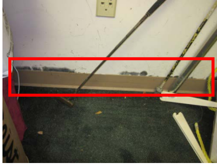
Mold-like substance found at base of interior wall
