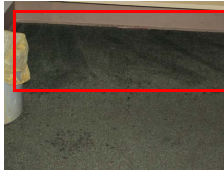
Wet carpet in corner of office area
