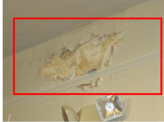
Damaged lath and plaster on interior wall section
