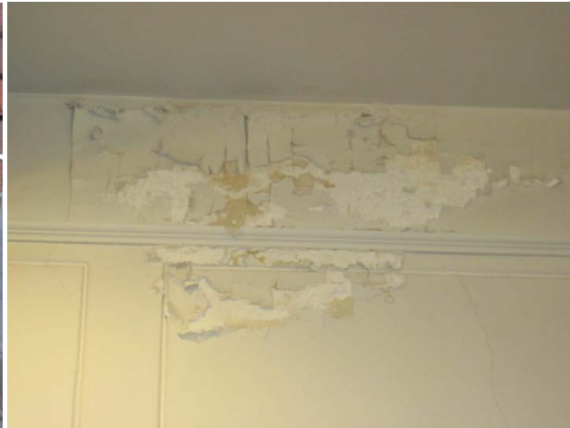
More damaged lath and plaster
