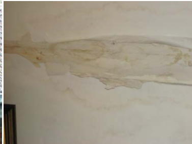
Damaged lath and plaster from water damage
