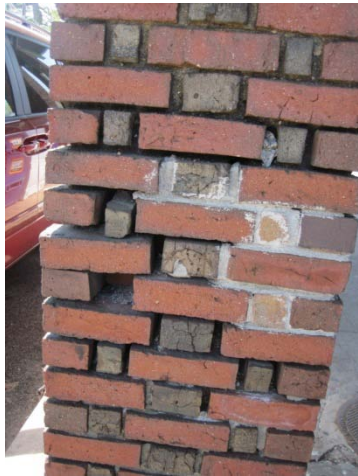
Mortar joints deteriorated
