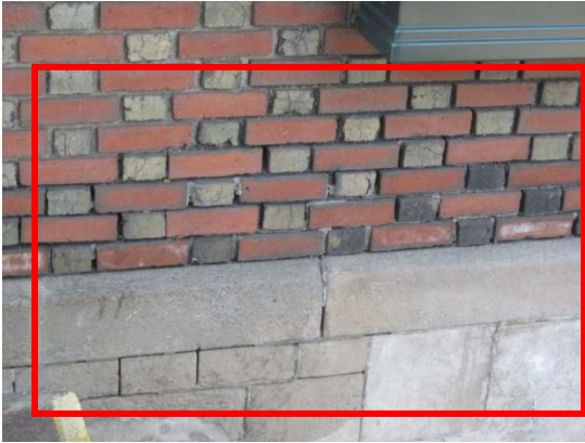
Deteriorated mortar joints due to water damage at perimeter walls and ineffective site drainage
