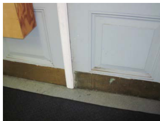
Un-insulated door with worn weather-stripping
