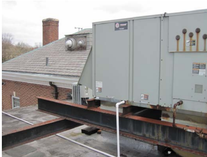
Rooftop packaged unit providing heating and cooling to building
