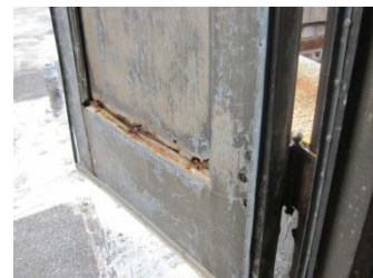
Damaged door leading to flat roof section
