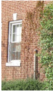
Overgrown ground vegetation growing on exterior wall surfaces
