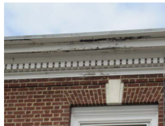
Chipped paint and potential wood rot due to water runoff
