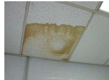
Damaged ceiling tile from plumbing leak or roof run off
