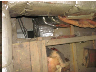
Duct chases permitting cold/hot attic air into conditioned building
