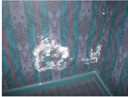
Interior wall damage showing moisture penetrating from exterior wall issue or roof run off compromising wall cavity
