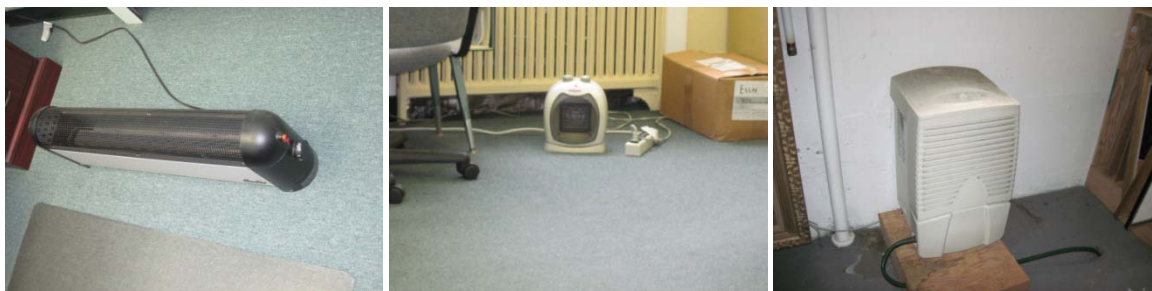
Space heaters found in various office areas; One of two dehumidifiers in basement
