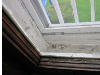
Single-glazed aged window with damaged frame
