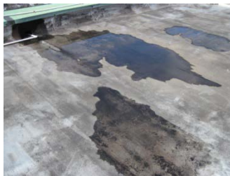
Signs of standing water/pooling
