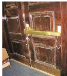
Un-insulated wood door
