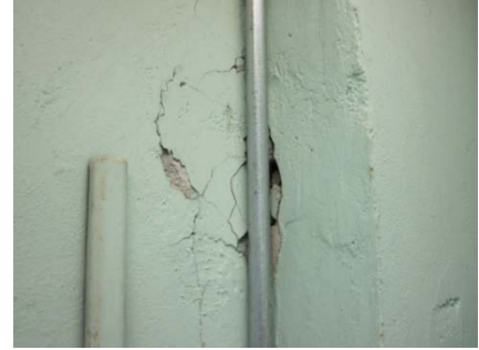
Damaged plaster wall section in basement
