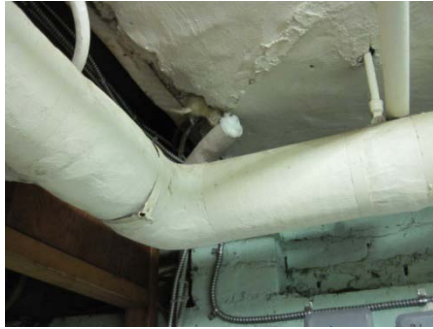
Asbestos-like substance found on piping in basement
