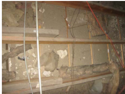
Bays between ceiling joists void of insulation
