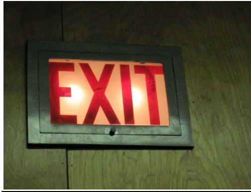
Exit sign found in court room
