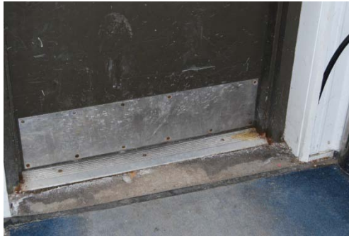
Damaged/warped/aged door frame
