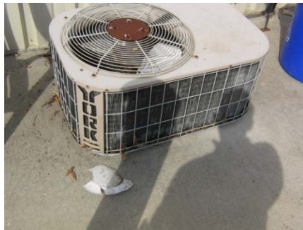
Split system condensing unit serving office area
