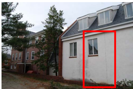
Mold/water damage on interior gypsum wallboard and exterior stucco finish due to uncontrolled water infiltration through the roof area.
