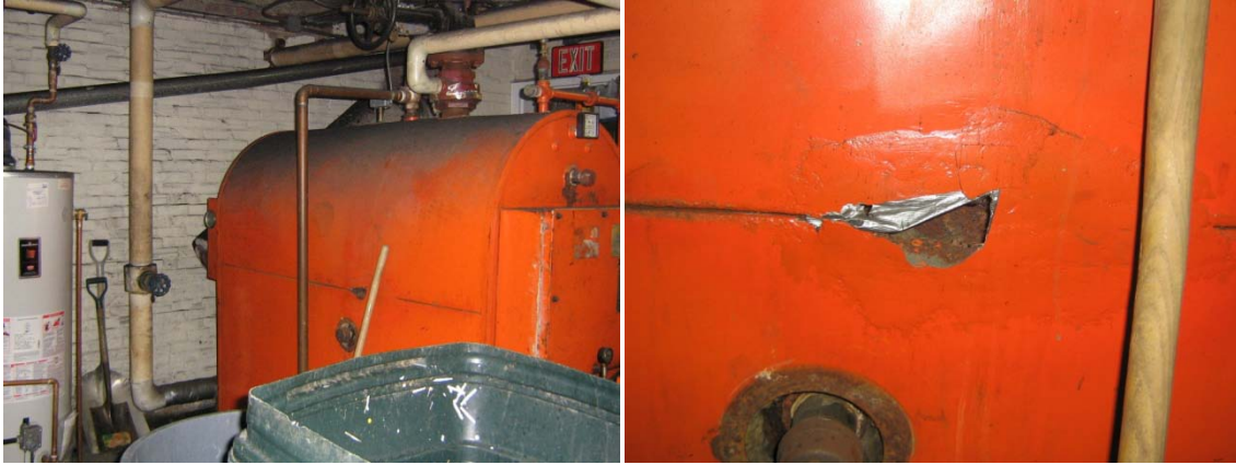
Oil -Fired Boiler and Photo of Hole in Outer Jacket
