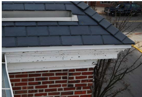
Deteriorating crown/fascia molding.
