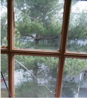
Single-glazed window with ineffective frame
