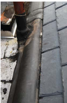
Rubber membrane instead of metal flashing installed with pocket for water and debris to collect and potentially leak into the building.
