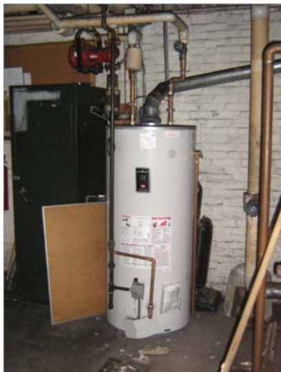
Gas-fired water heater
