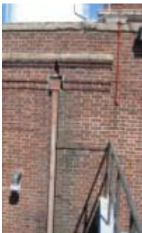
Uncontrolled roof water run-off due to defective gutters, downspouts and flashing.
