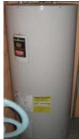
Bradford White water heater
