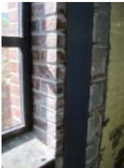
Efflorescence on brick and masonry walls indicate moisture presence within the wall cavity.
