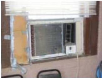
Air-leakage at sleeved window/wall air-conditioning
