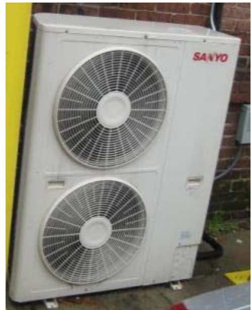
Figure 2: Sanyo split-system condensing unit
