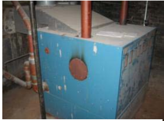
Figure 1: Burnham steam boiler
