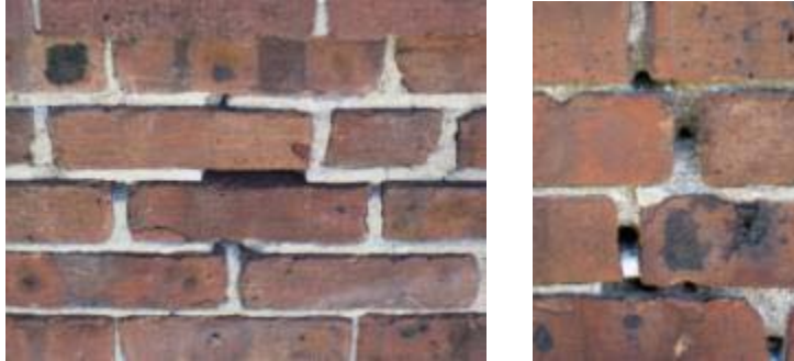
Cracked/deteriorated mortar joints were detected
