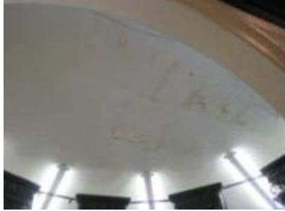
Signs of water damage on interior finishes due to flat roof leak above.
