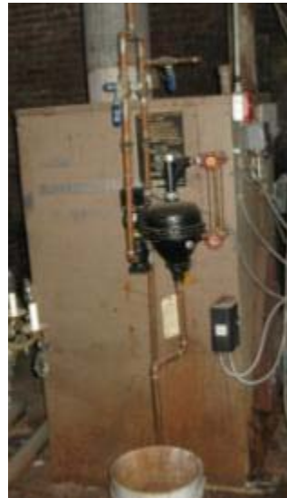
Figure 1: American Standard steam boiler
