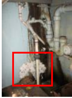
Deteriorating interior wall finishes due to moisture exposure
