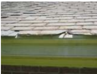
Cracked/missing slate tiles
