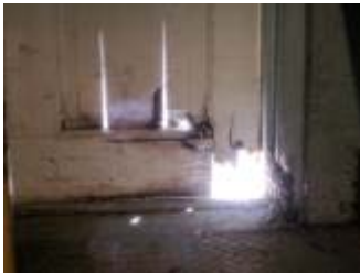
Damaged door and frame
