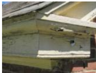
Deteriorating exterior wood crown trim and returns.
