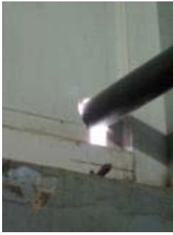
Un-caulked/un-sealed exterior wall penetrations
