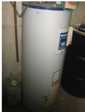
Domestic Water Heater
