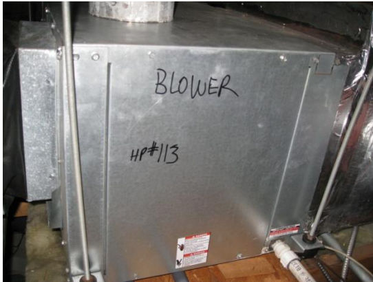
Typical Fan in Attic Used for Supply or Exhaust Air
