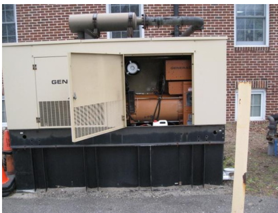
Emergency Generator at Rear of Building
