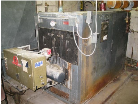
Hot Water Boiler
