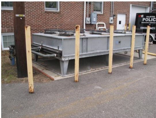
Fluid Cooler at Rear of Building
