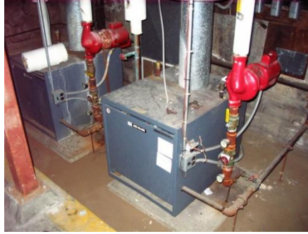
Gas-fired Boilers in Basement Mechanical Room
