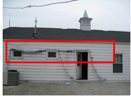
Interaction between electrical cable and exterior wall finish could lead to an unsafe situation
