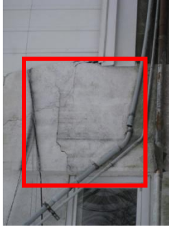
Cracked or deteriorating stucco showing signs of water/moisture
