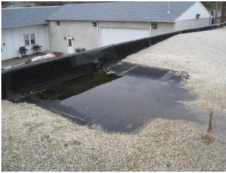
Water pooling on side of the flat roof
