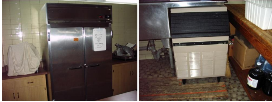
Commercial Refrigerator (left) and Ice Machine in Kitchen
