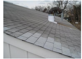
Old backside asphalt shingle roof
