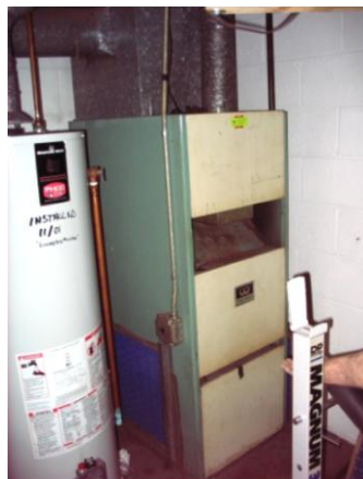
Domestic Water Heater and Furnace in Small Gym
