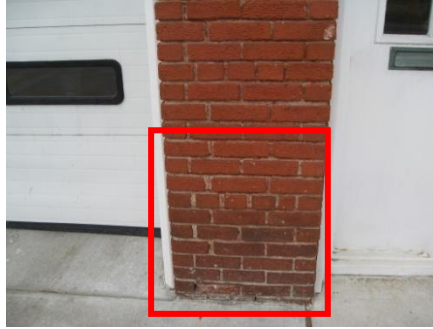
Deteriorating exterior wall finish in need of brick re-pointing
