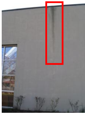
Uncontrolled roof water run-off due to missing gutters and downspouts - Library
