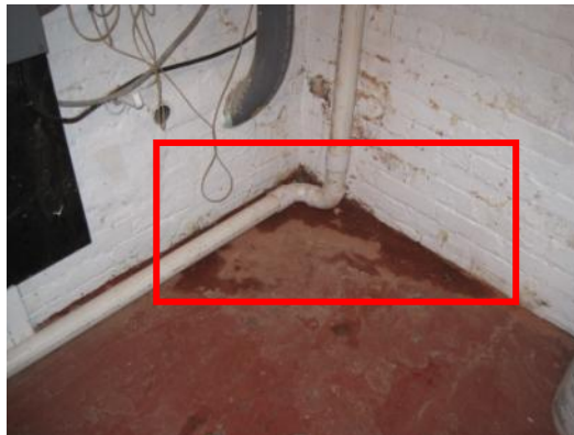
Water/moisture seepage through cracks detected in the slab in Borough Hall pump room
