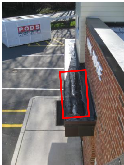
Signs of standing water/pooling
