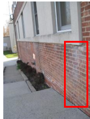
Efflorescence on brick and masonry walls indicate moisture presence within the wall cavity- Borough Hall.
