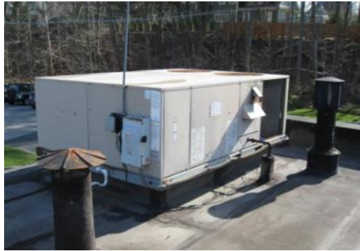
Public Library Roof: Old Luxaire Rooftop Unit
