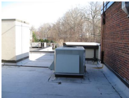
Central Corridor Roof: Trane Rooftop Unit
