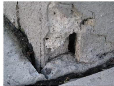
Damaged EIFS – Library
