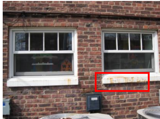
Exterior mold/water damage signs on areas around windows- Borough Hall
