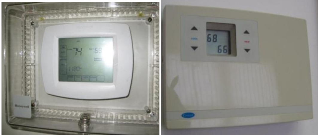
Typical Programmable Thermostat for 13 zones (left); Damper Controls for Offices based on temperature (Right)
