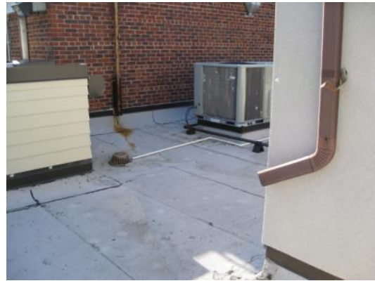
Drainage from second floor roof to first floor roof above connection area between Borough Hall and Public Library
