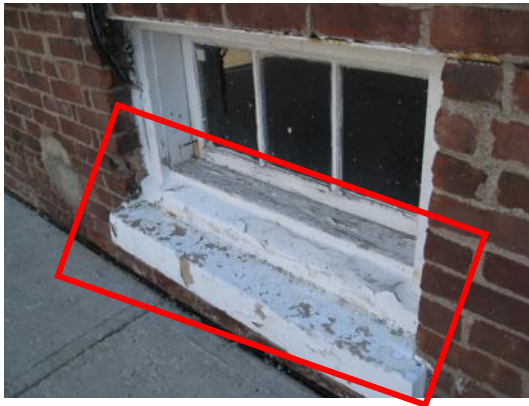
Damaged/aged window frame – Borough Hall
