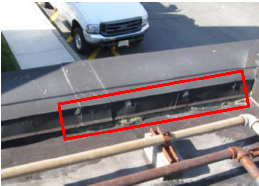
Uncontrolled vegetation growth on roof of Public Library
