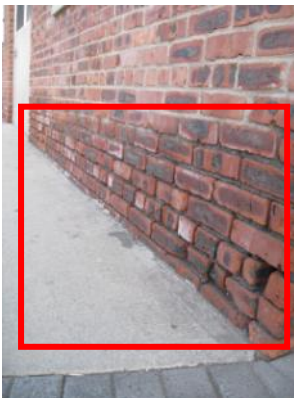
Cracked/deteriorated brick and mortar joints – Borough Hall
