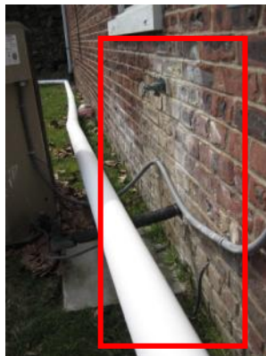
Efflorescence on brick and masonry walls indicate moisture presence within the wall cavity- Borough Hall.
