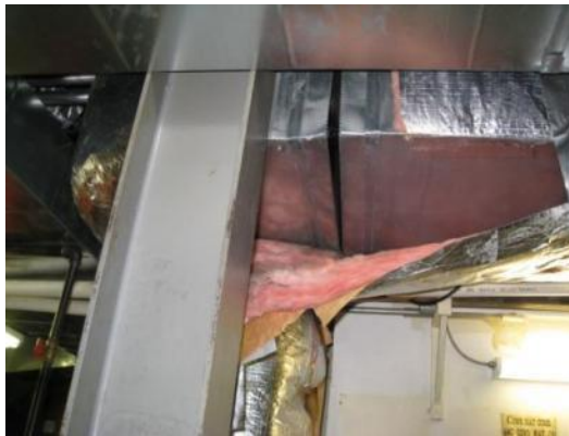
Damaged insulation on ductwork in Borough Hall Mechanical Room
