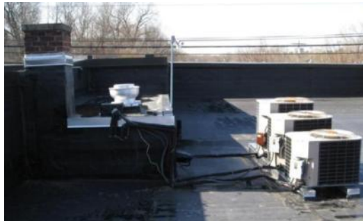
Borough Hall Roof: Three Luxaire condensers with insulated refrigerant pipes leading to building furnaces
