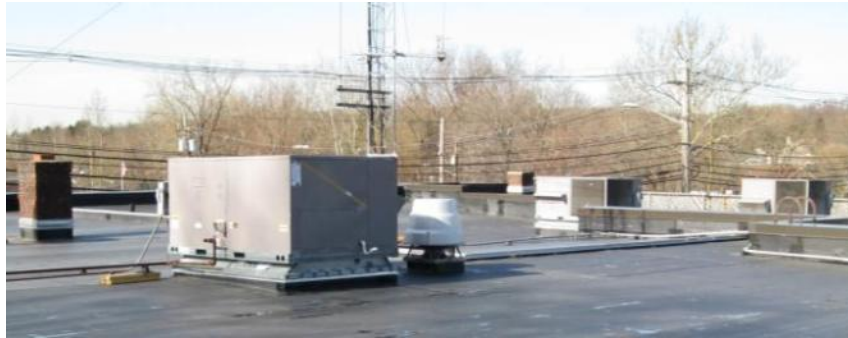
Rooftop units, fans and chimneys on Borough Hall new EPDM flat roof
