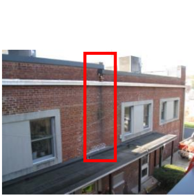
Uncontrolled roof water run-off due to missing gutters and downspouts – Borough Hall
