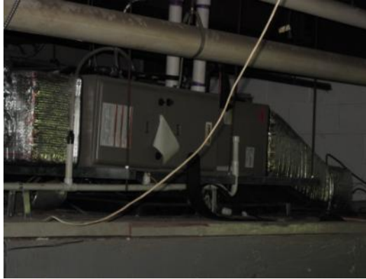
Break Room Condensing Furnace
