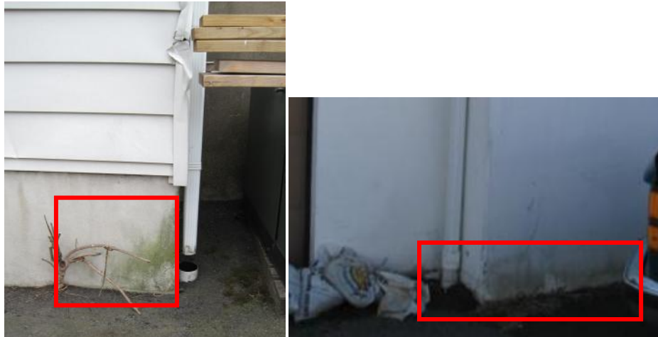
Potential water/moisture seepage through vegetation growth detected at the slab
