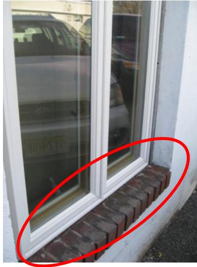
Exterior mold/water damage signs on areas around windows
