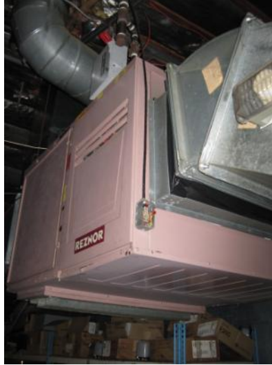
Reznor 100% Outside Air Ventilation Unit
