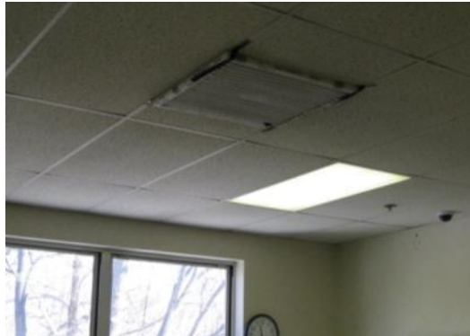
Air Supply grill covered with filter in 2 nd Floor Office
