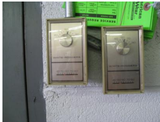
Unit heater manual thermostats
