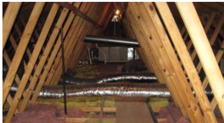
Insulated round ductwork for second floor office supply air
