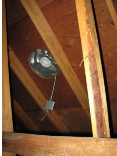
Installed but disconnected attic exhaust fan
