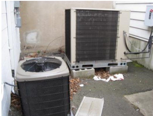
Outside condensing unit to disperse heat to atmosphere
