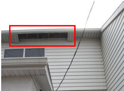
Missing eave vent panels on second floor
