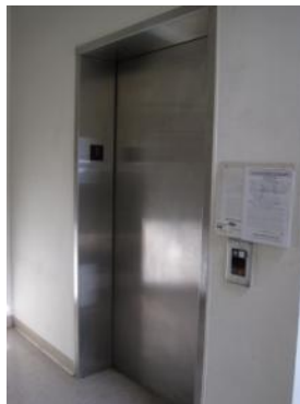
Elevator in lobby
