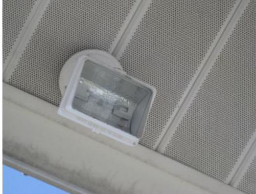
Exterior Metal Halide Fixture
