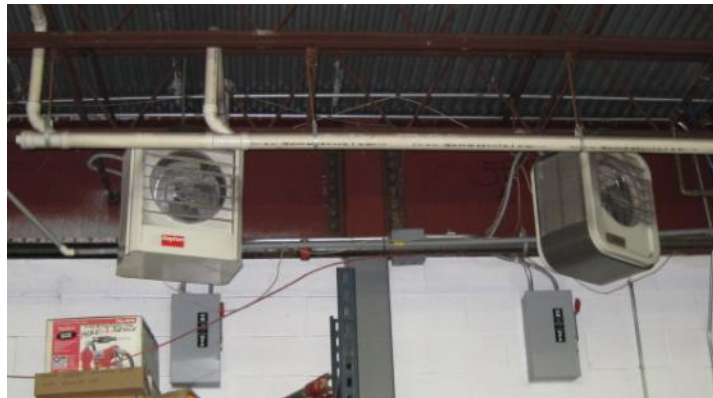
Qmark and Dayton Electric Unit Heaters in Garage
