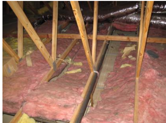
Uneven attic insulation found
