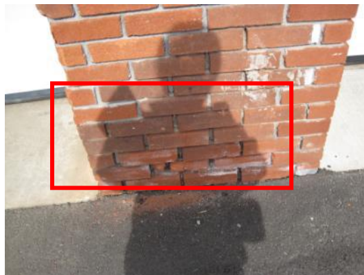
Cracked/deteriorated mortar joints on brick veneer, near base
