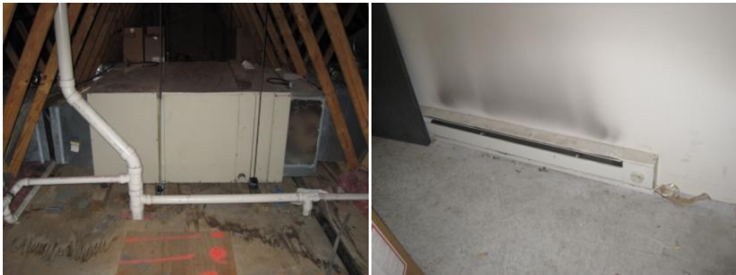
Lennox Condensing Furnace and Electric Baseboard Heaters
