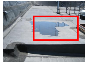
Signs of standing water/pooling
