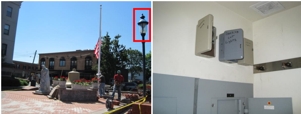
Parking lot pole lights and timers controlling entry doors, parking and canopy lights
