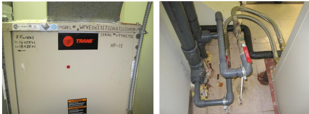
Typical water source heat pump and associated cooling water supply/return piping
