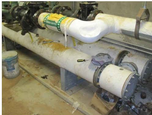
Heat exchanger to remove heat rejected by heat pumps with cooling tower water
