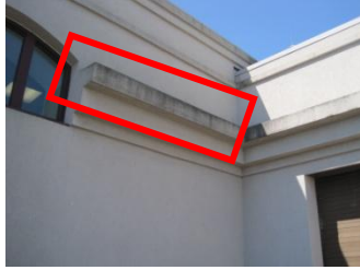
Uncontrolled roof water run-off due to missing gutters and downspouts
