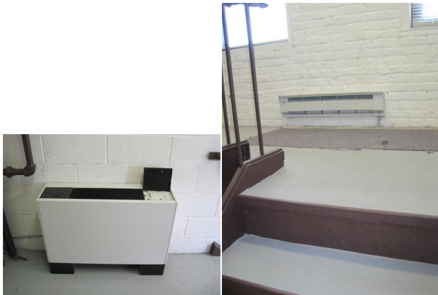
Stairwell cabinet and baseboard electric unit heaters
