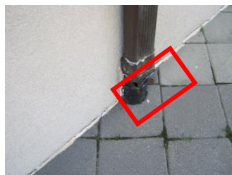
Water/moisture seepage through joints at slab and worsened by cracked downspout connection
