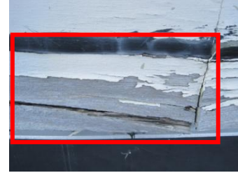
Missing/deteriorating wood trim
