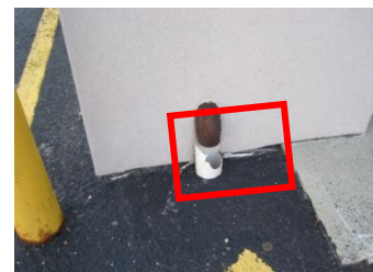
Water/moisture seepage through joints at slab and worsened by cracked downspout connection
