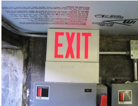
Typical LED Exit sign - 5 Watt lamp
