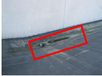
Signs of standing water/pooling
