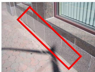
Water/moisture seepage through joints at the slab
