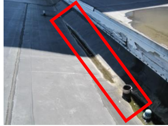
Signs of standing water/pooling
