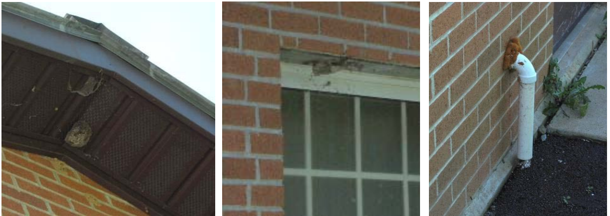
Insect nesting around eaves and windows in addition to inappropriate wall penetration sealer were found
