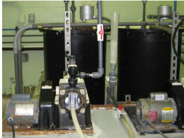
Two (2) chemical feed pumps
