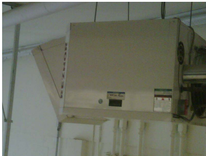
Typical Reznor unit heater found in garage area
