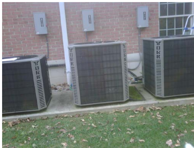
Condensing units located outside the building
