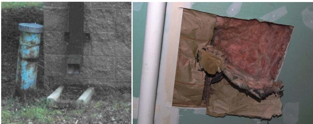
Downspout diverter with insufficient slope Unsealed openings in ceiling
