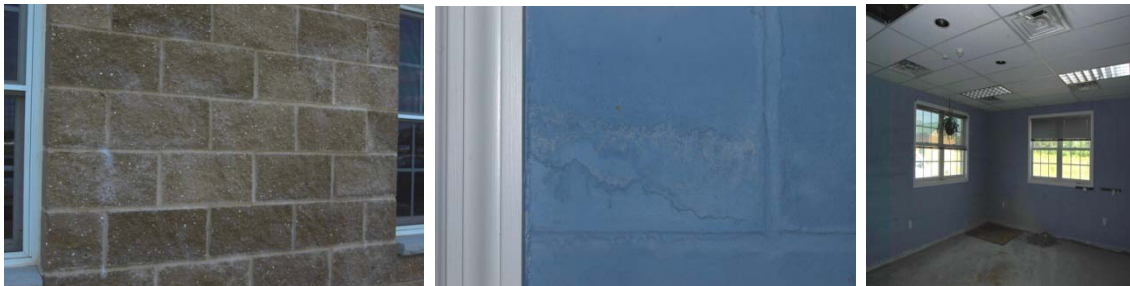
Efflorescent and other water problems visible on the interior and exterior walls
