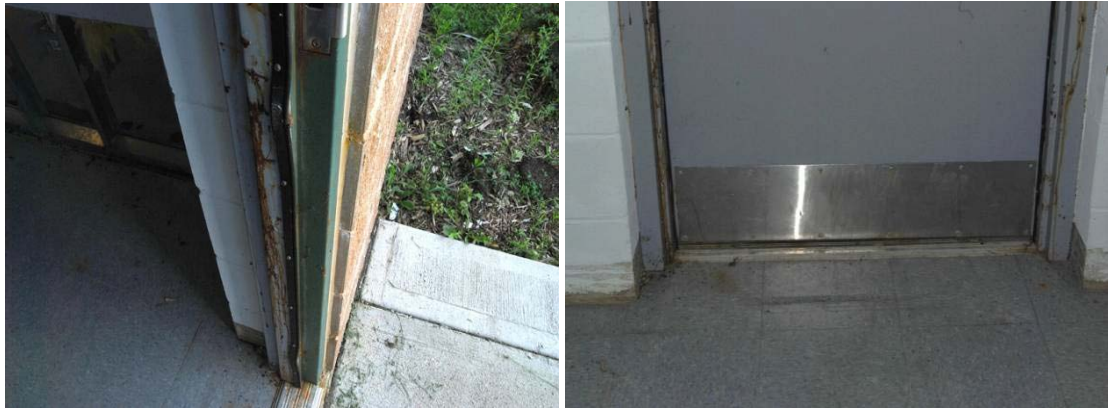
Worn and missing weather stripping around doors
