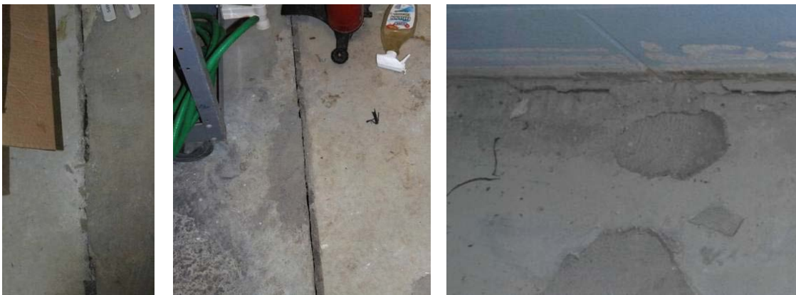
Signs of differential settlement in slab
