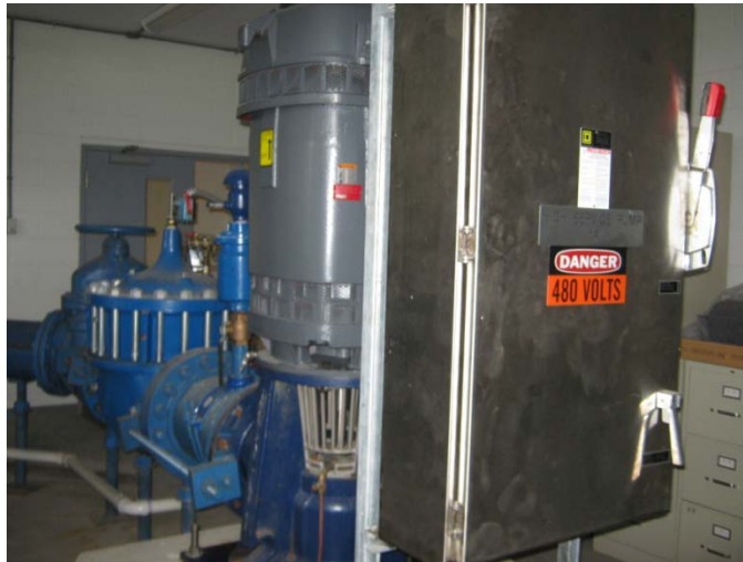
Pumps and motors located at Germany Flats
