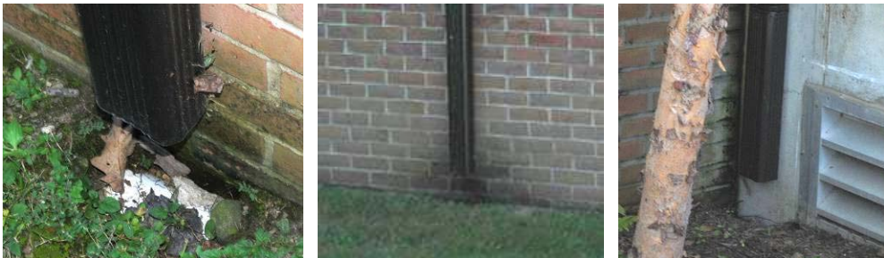
Downspout deflectors and diverter missing, causing water penetration between basement wall and insulation
