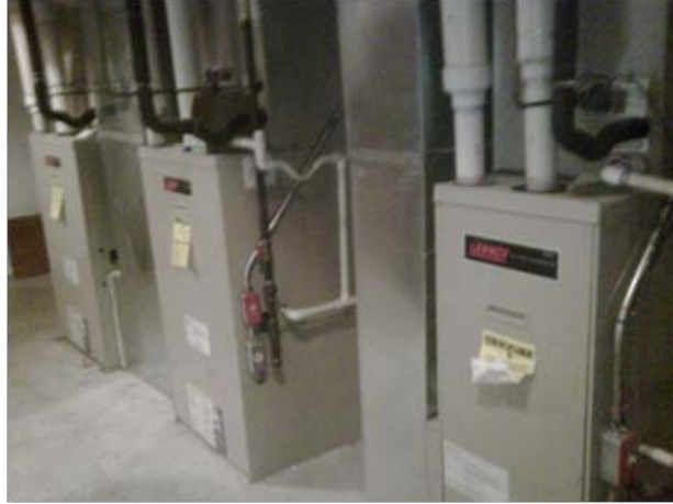
Sample of heating furnaces
