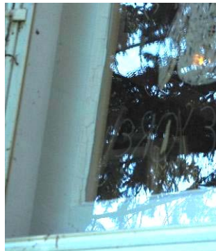
Original single pane windows with cracked panel
