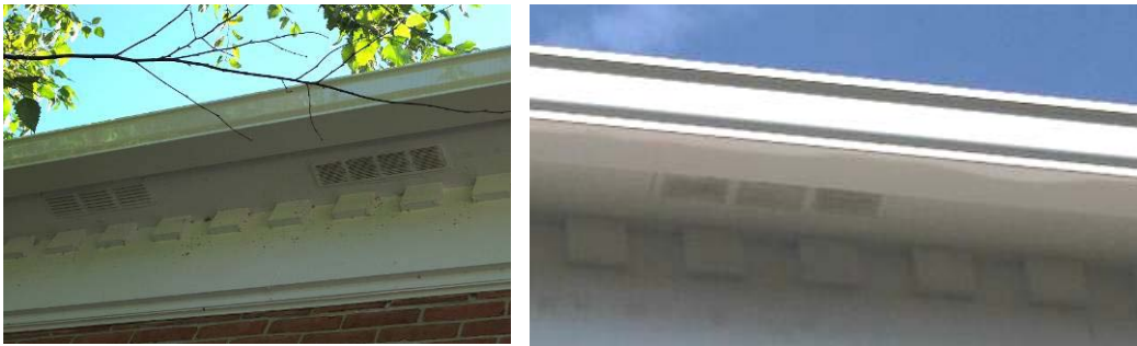
Insufficient amount of soffit vents
