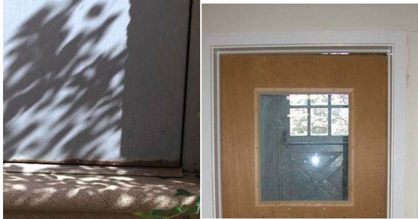
Worn and missing weather stripping around doors.
