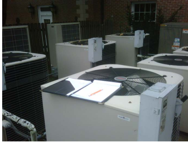
Condensers located outside along the exterior wall of the building
