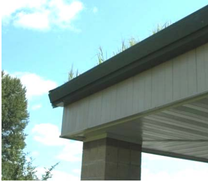
Gutters in need of cleaning
