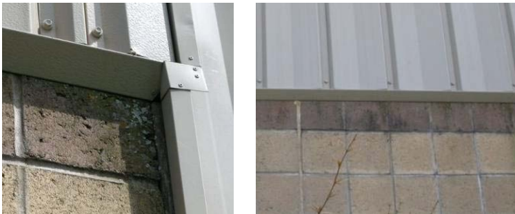
Water penetration due to flashing problems at metal panel terminations
