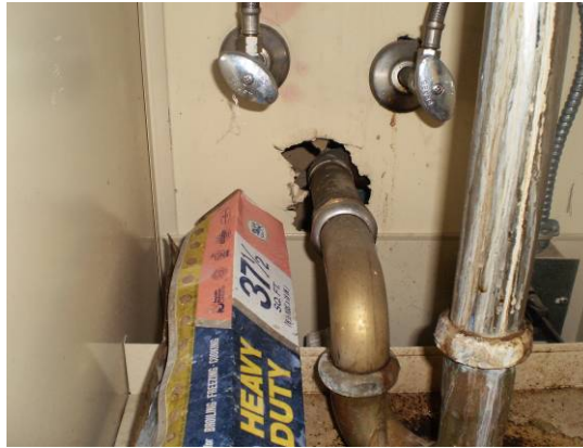
Piping penetrations under sink in meeting room
