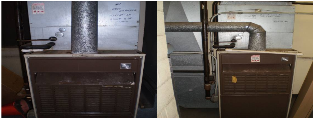
Furnace Units #1 and #2 (Typical furnace units)
