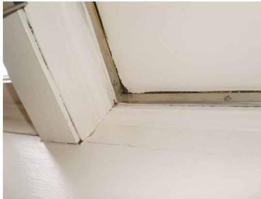
Edges of door in Public Assembly room no longer form tight seal
