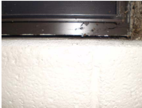
Poorly sealed window located in sign shop
