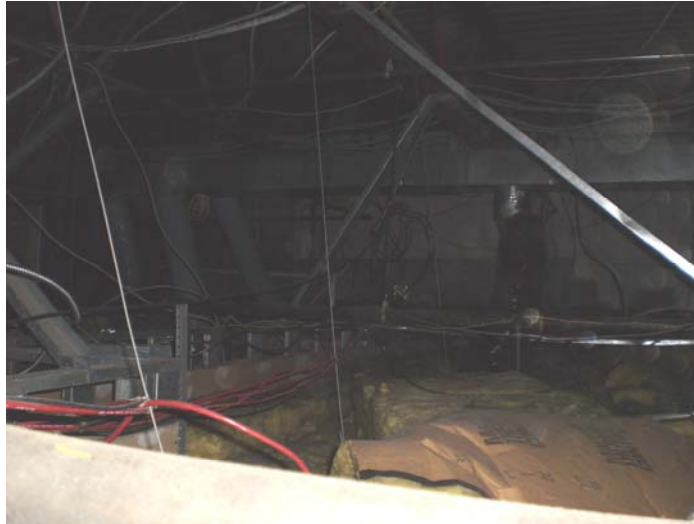
Plenum above office – batt insulation is compressed and out of place
