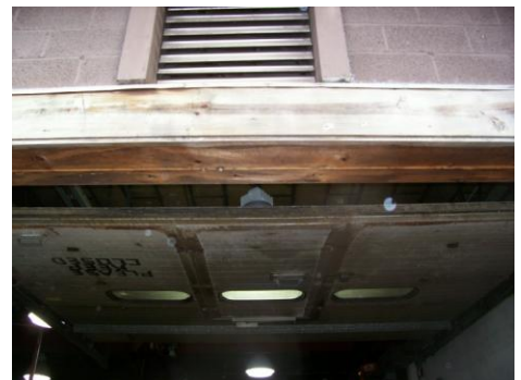
Door showing worn weather stripping and over-head type door without a base gasket
