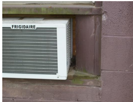
Window air conditioning unit found without proper seals and gaskets
