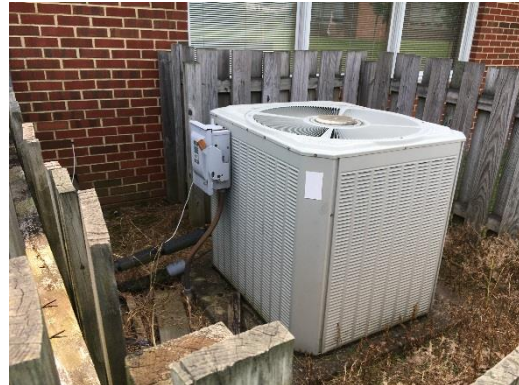
AHU Systems – Outdoor Condensing Unit
