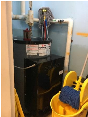
Storage Tank Water Heater
