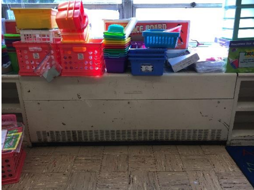
Original Unit Ventilator
