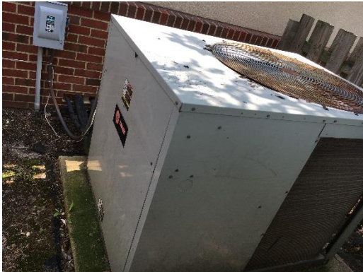
AHU Systems – Outdoor Condensing Unit
