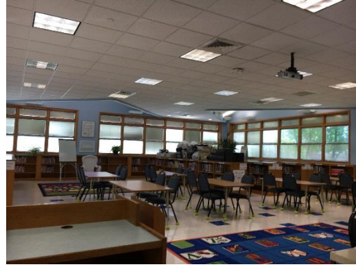
Media Center Lighting
