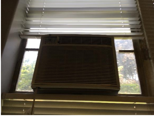
Window AC Unit
