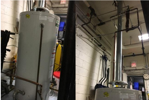
Storage Tank Water Heater and Uninsulated Piping
