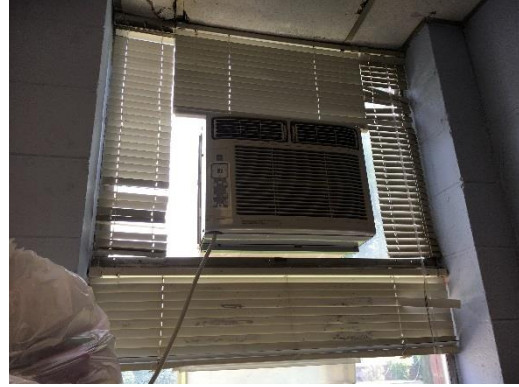
Window AC Unit
