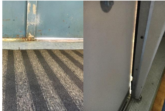
Exterior Doors with Worn Weather-Stripping
