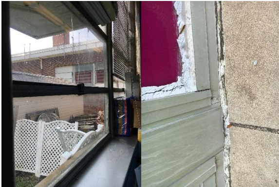
Building Envelope Deficiencies
