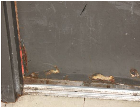
Exterior door needing replacement
