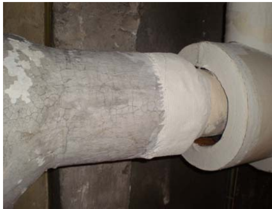
Asbestos insulation on piping
